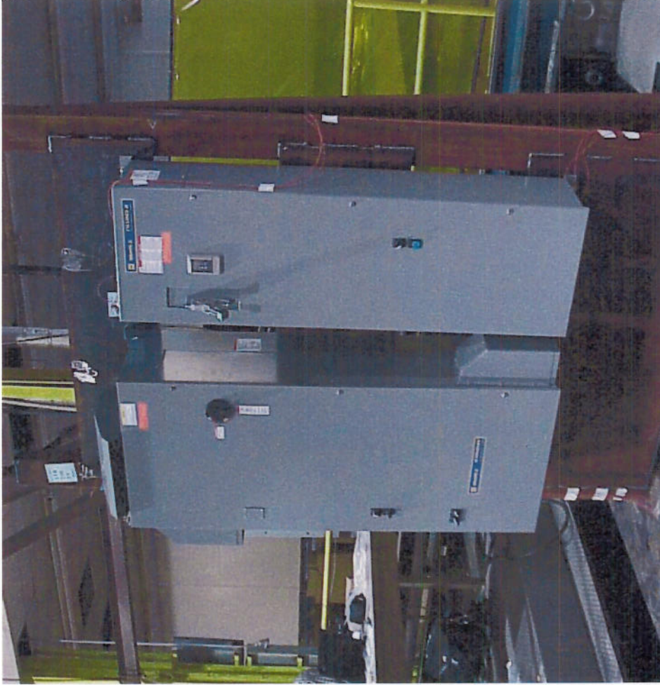
UUT1 - ATS 48 (Right) UUT2 - Drive 8839 (Left)
