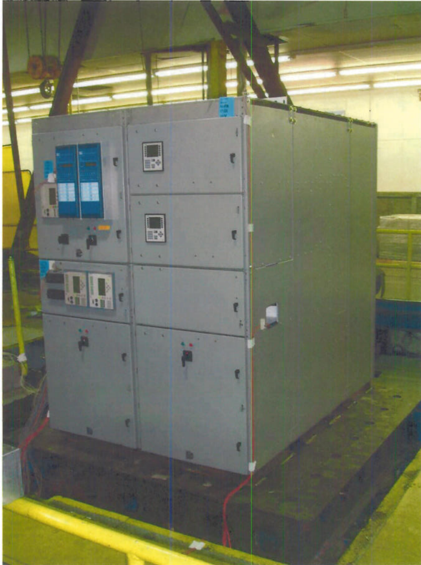
15 KV Medium Voltage Switchgear
