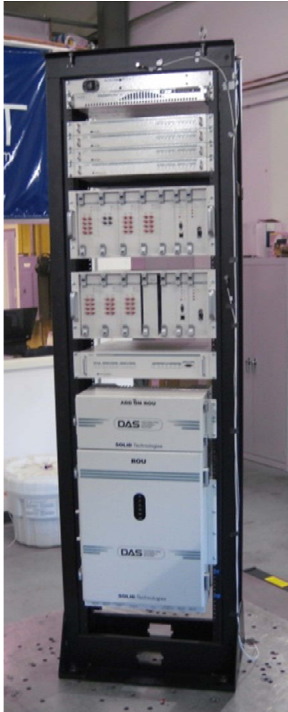
UUT 11, 2-Post Rack with Alliance Components
