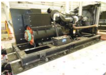
Figure 1: UUT-5A 400kW Generator on shake table Anchorage: Base bolted to plates w/ (10) 5/8" dia Grade 8 bolts
