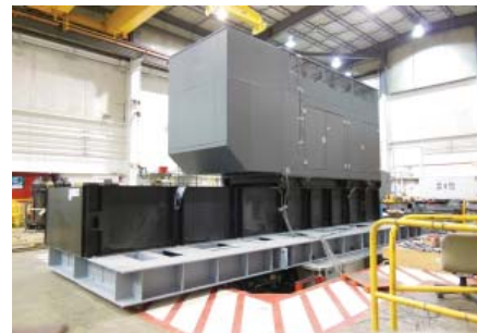
Figure 4: UUT-6B/6C 600kW Generator w/ enclosure and fuel tank Anchorage: Unit Base bolted to tank w/ (12) 5/8" dia Grade 8 bolts Tank bolted to fixture w/ (18) 3/4" dia Grade 8 bolts
