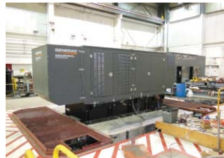
Figure 2: UUT-5B/5C 400kW Generator w/ enclosure and fuel tank Anchorage: Unit Base bolted to tank w/ (10) 5/8" dia Grade 8 bolts Tank bolted to plates w/ (10) 5/8" dia Grade 8 bolts
