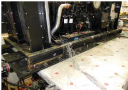
Figure 3: UUT-6A 600kW Generator on shake table Anchorage: Base bolted to plates w/ (12) 5/8" dia Grade 8 bolts
