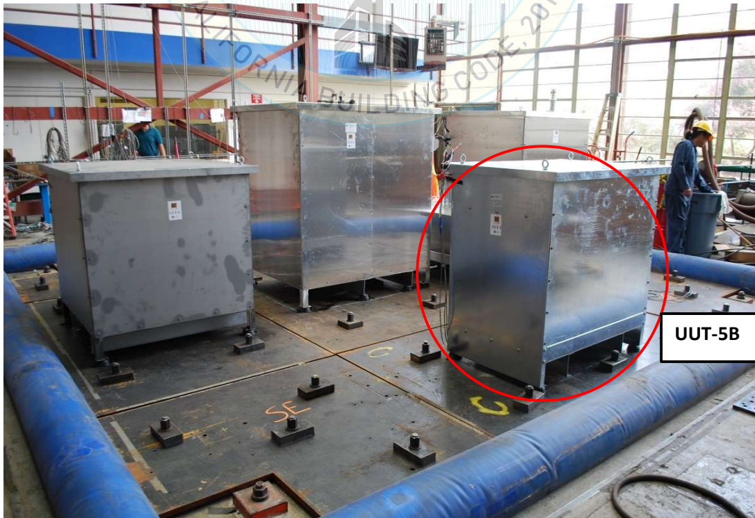
All units were filled with contents and maintained structural integrity and functionality after AC-156 test.
