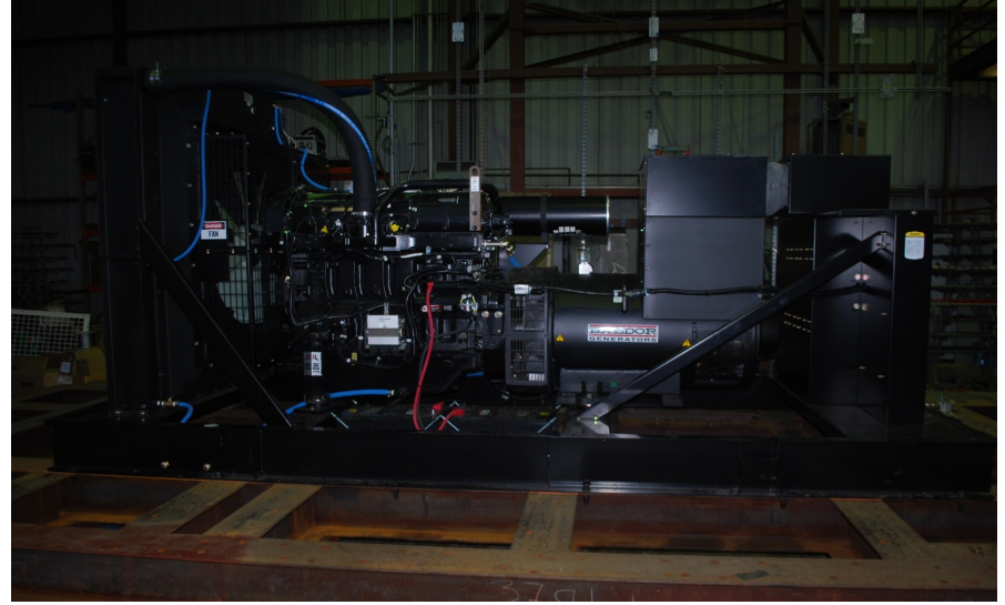
UUT 4C Genset Skid is Mounted Directly to the Fixture Using (12) 3/4" Diameter ASTM A490 Bolts.
