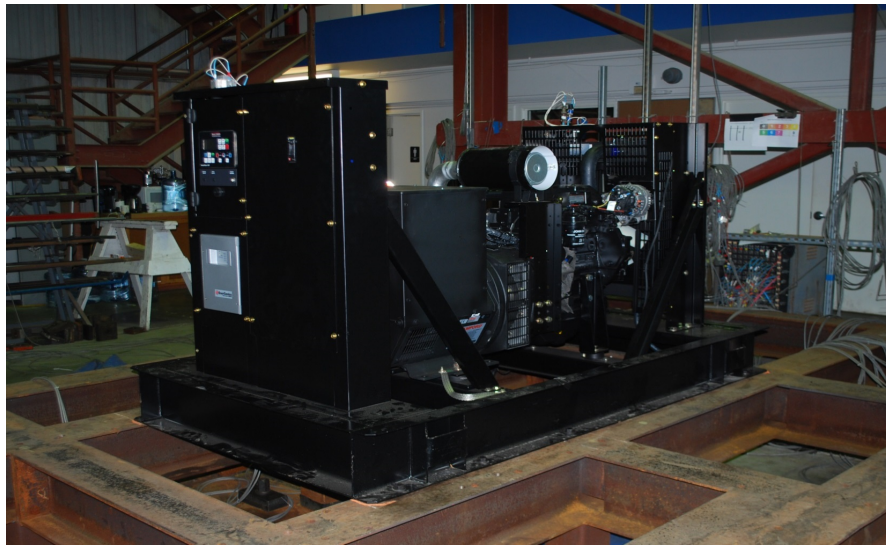
UUT 2C Genset Skid is Mounted Directly to the Fixture Using (12) 3/4" Diameter ASTM A490 Bolts.
