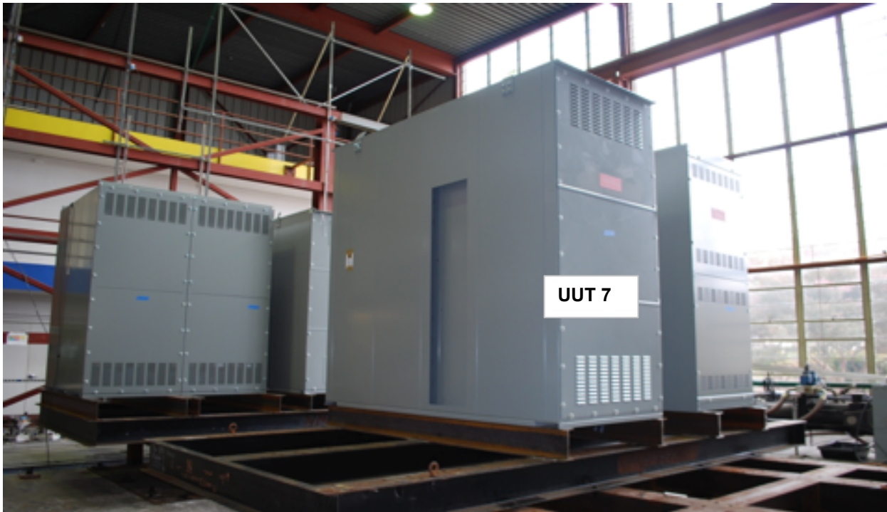
All units were filled with contents and maintained functionality and structural integrity
