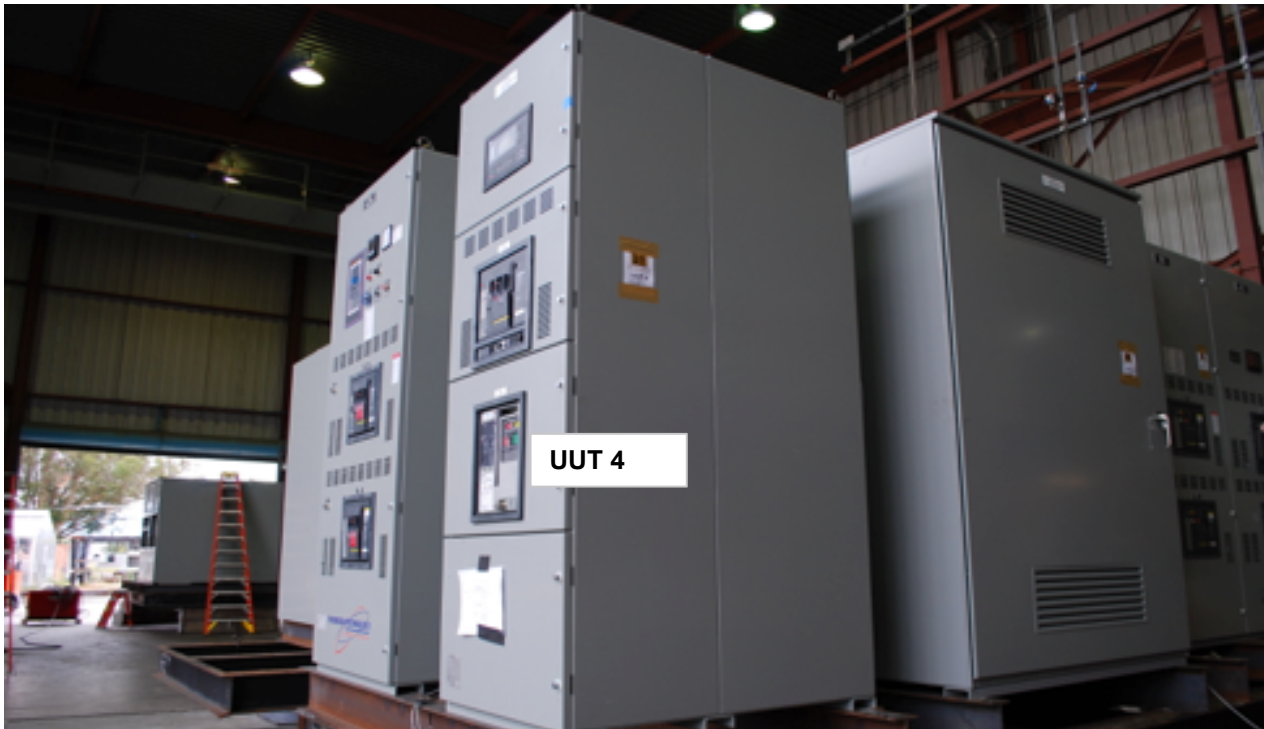
All units were filled with contents and maintained functionality and structural integrity
