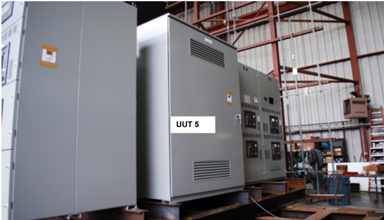
All units were filled with contents and maintained functionality and structural integrity
