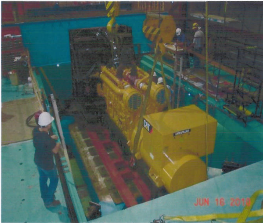
C3516 Mounted onto The VMC Group M2SSH Isolators
