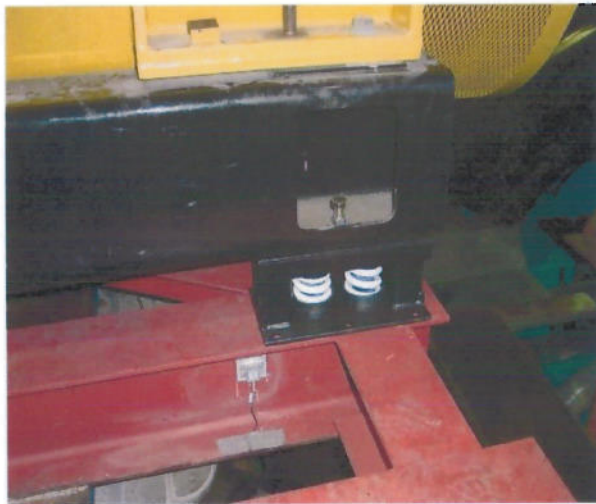
Unit Mounted onto The VMC Group M2SSH Isolators
