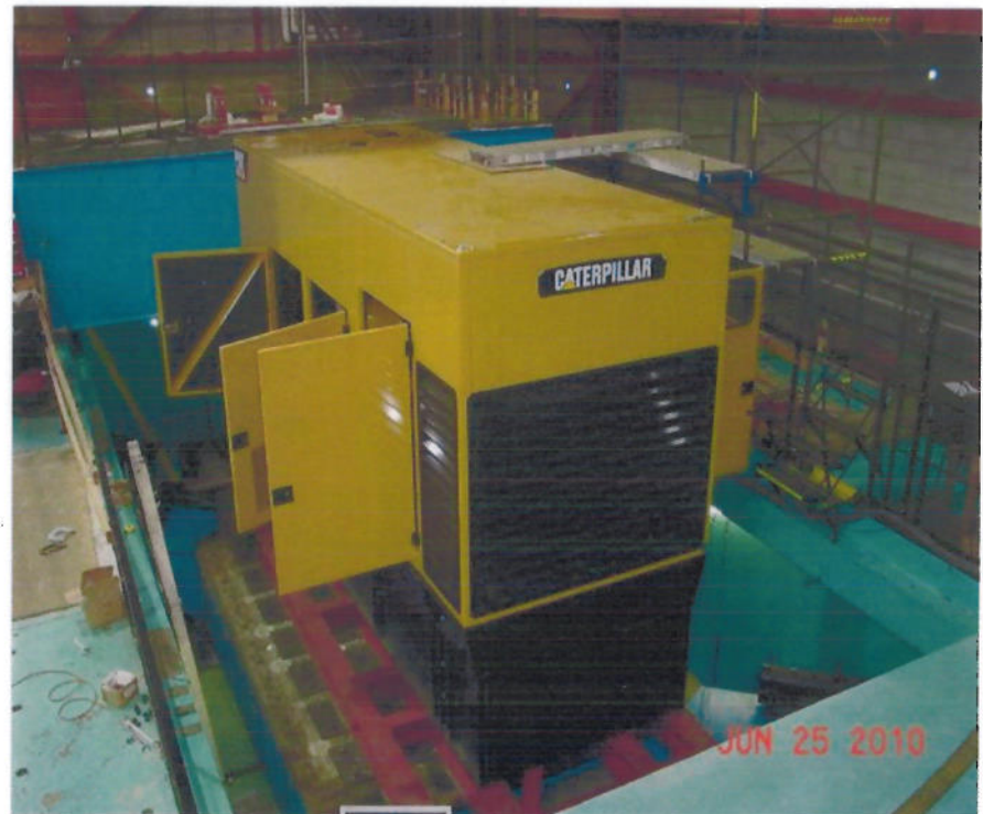
Enclosed C27 Mounted on UL142 Fuel Tank
