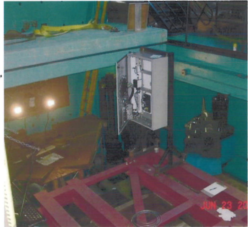
Control Panel Mounted to Structural Fixture
