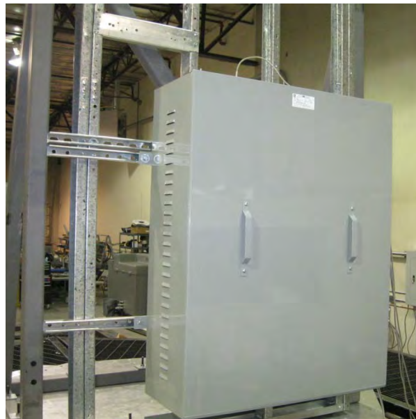
UUT3, wall-mounted to shake table interface frame.
