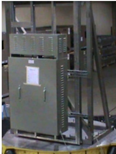
UUT2, wall-mounted to shake table interface frame.
