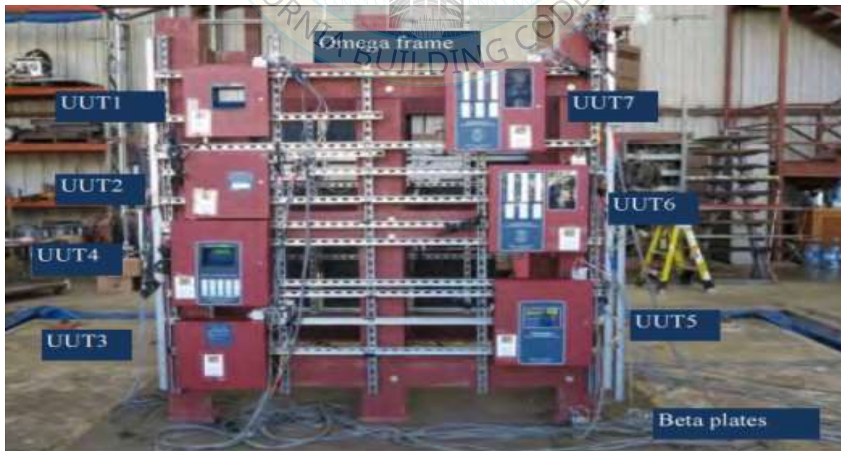
All units were filled with contents and maintained structural integrity and functionality after AC-156 test.
