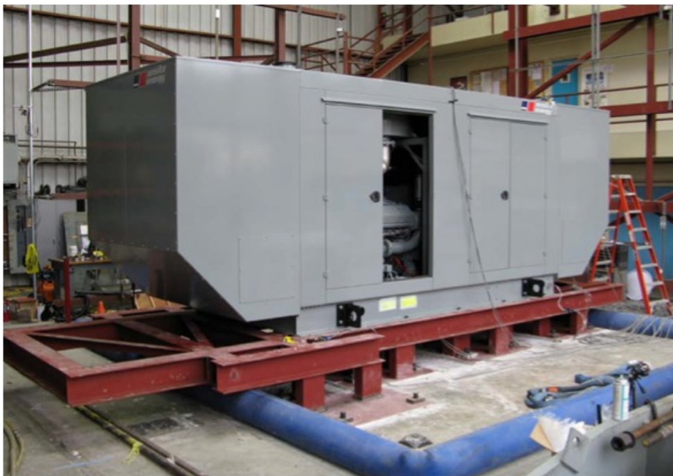
All units were filled with contents and maintained structural integrity and functionality
