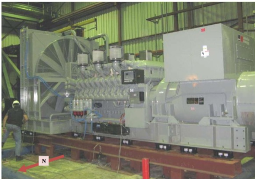
All units were filled with contents and maintained structural integrity and functionality
