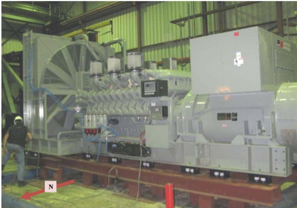
All units were filled with contents and maintained structural integrity and functionality
