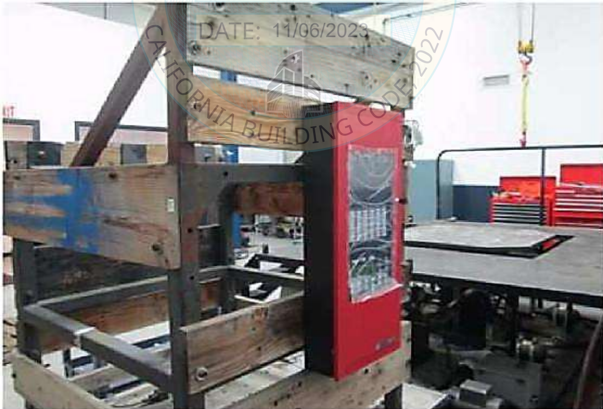
UUT-1 Overall View
