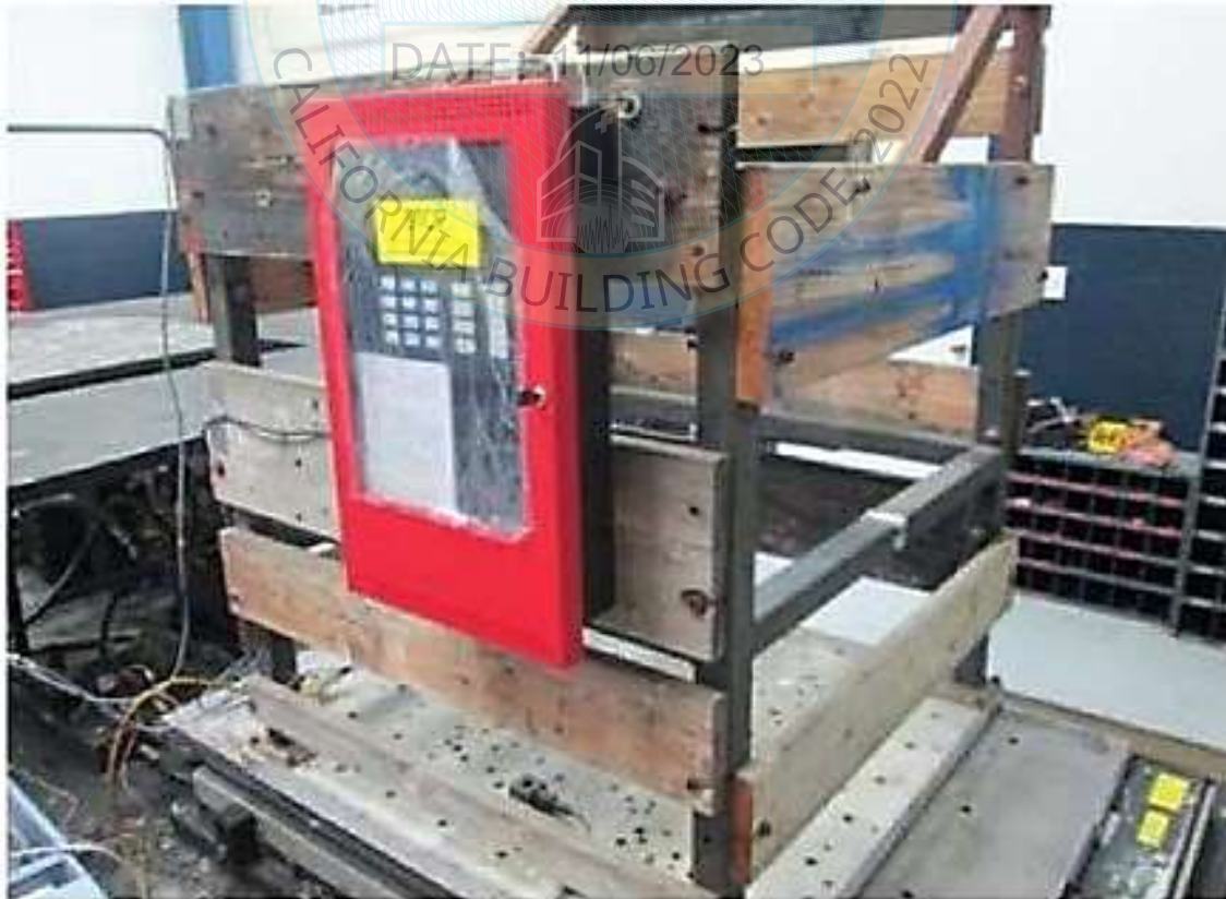
UUT-2 Overall View
