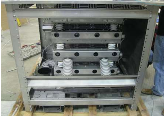
Side panels removed to photograph interior. Notice seismic bracing has been removed and number of insulators have been reduced.
