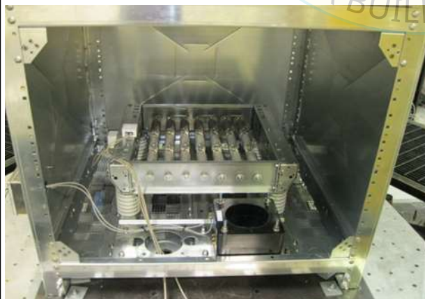
Side panel removed to photograph interior. Notice seismic bracing has been removed and number of insulators have been reduced.
