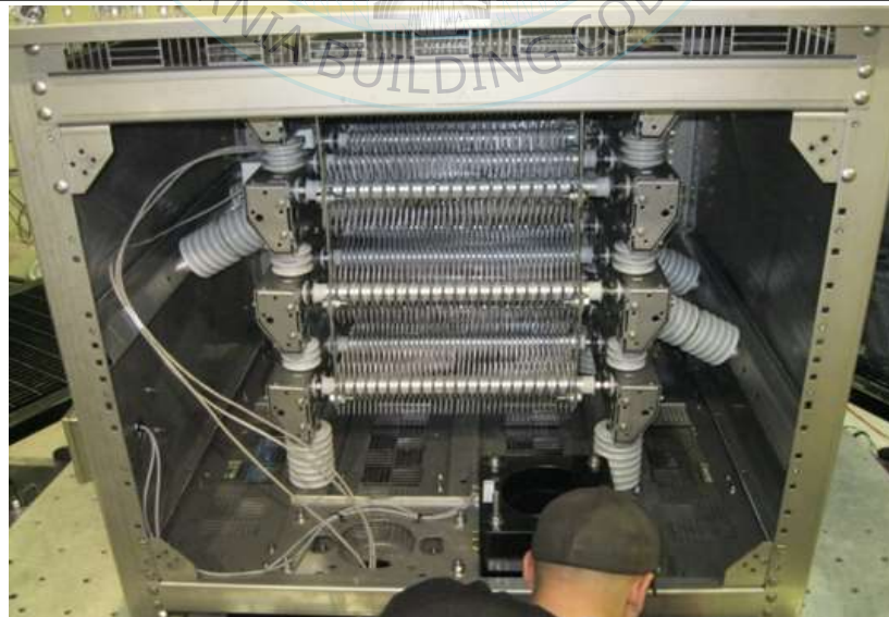
Side panel removed to photograph interior. Notice seismic bracing has been removed and number of insulators have been reduced.
