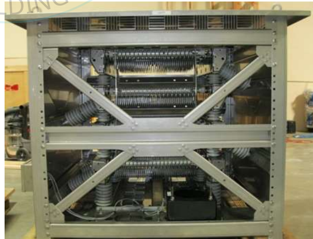
Side panel removed to photograph UUT1A interior.
