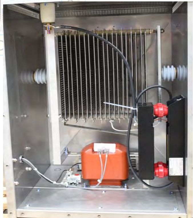
UUT-07B interior view.
