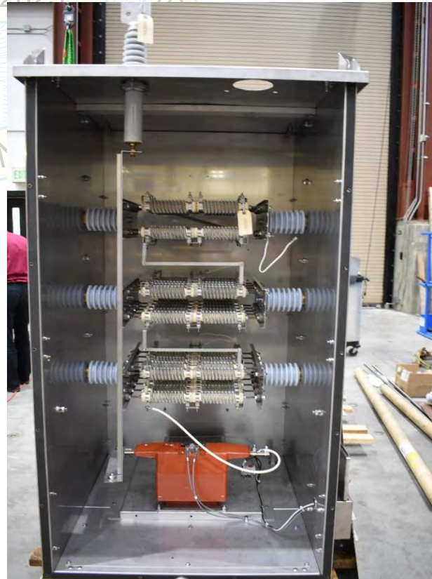
UUT-05B interior view.
