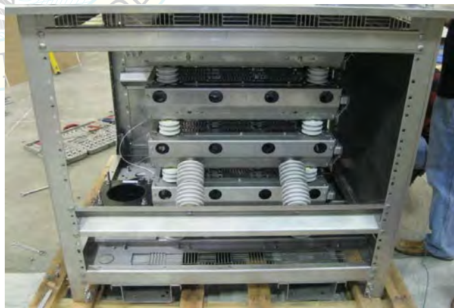
UUT-02B interior view.
