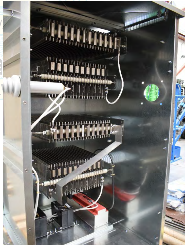
UUT-06A interior view.
