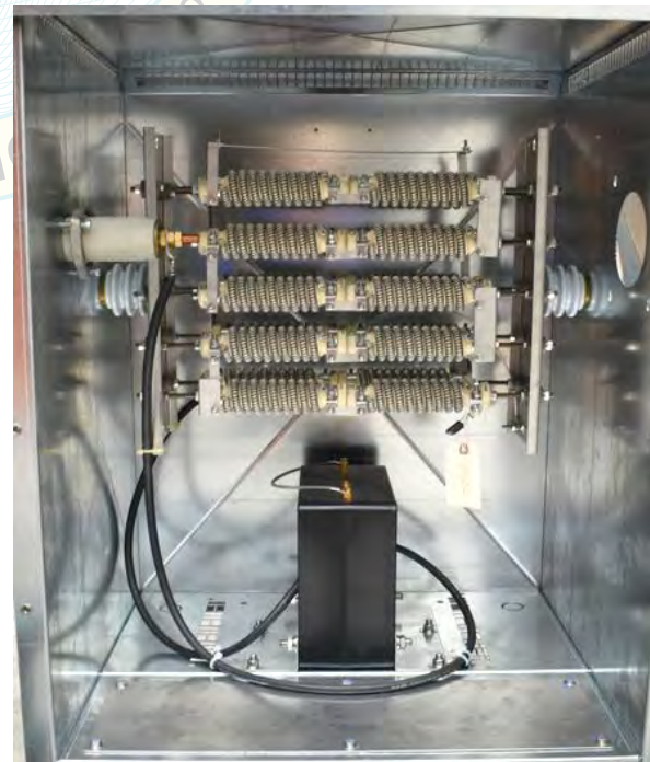
UUT-08A interior view.
