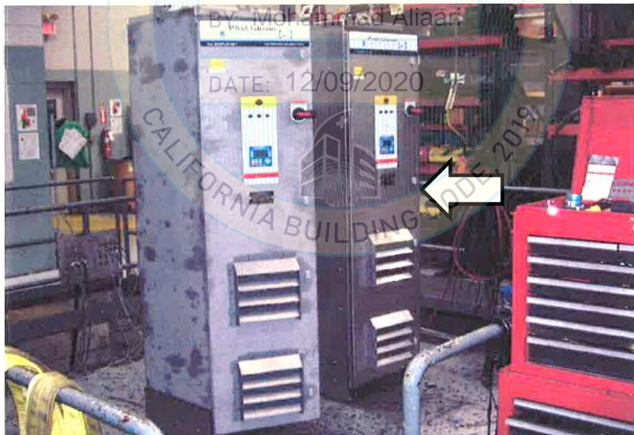
Photo of test setup (UUT2 is on the right)
