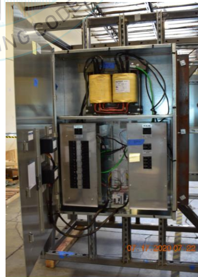
Figure 2. Interior View of UUT7
