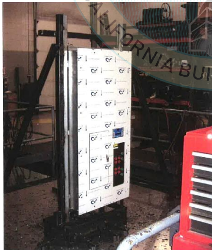
Figure 1. Exterior View of UUT1
