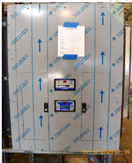
Figure 1. Exterior View of UUT6
