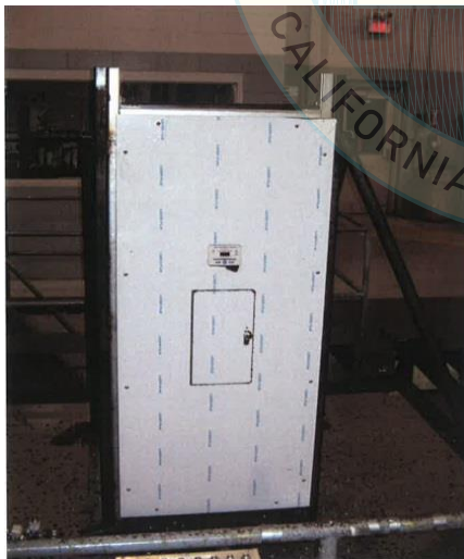
Figure 1. Exterior View of UUT3
