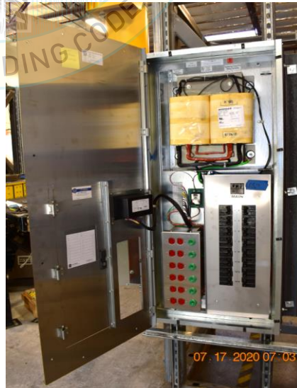
Figure 2. Interior View of UUT5
