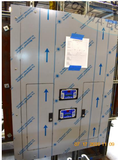
Figure 1. Exterior View of UUT7
