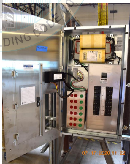
Figure 2. Interior View of UUT4
