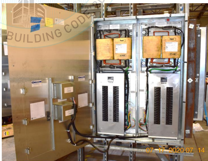
Figure 2. Interior View of UUT6
