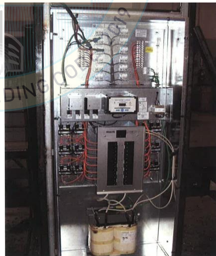
Figure 2. UUT3 Overall View with Front Panel Removed
