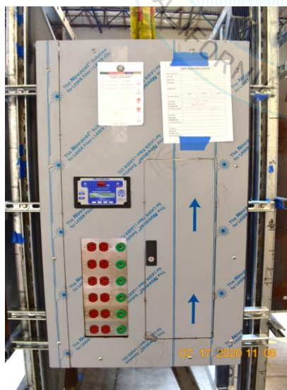
Figure 1. Exterior View of UUT4
