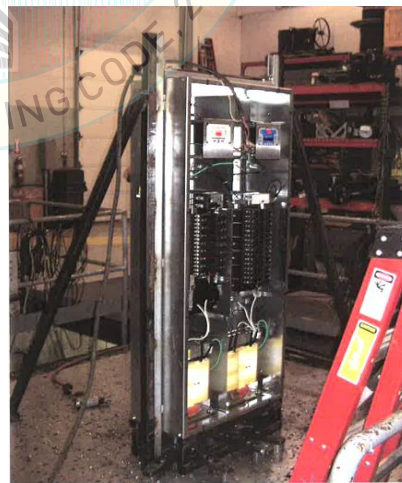
Figure 2. UUT2 Overall View with Front Panel Removed
