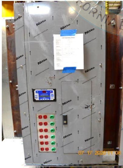
Figure 1. Exterior View of UUT5
