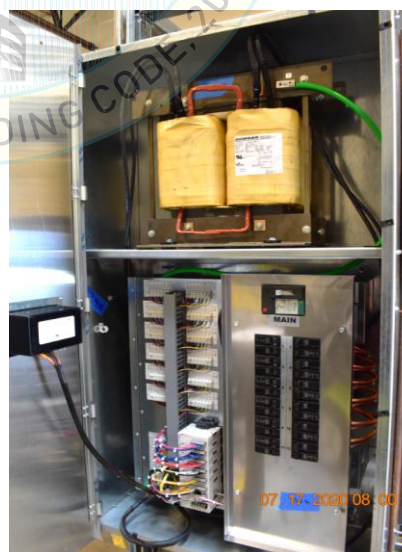
Figure 2. Interior View of UUT8
