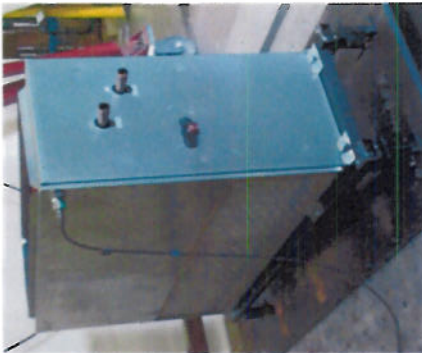
VEY20, Base Mounted on AMSR-1C Isolators
