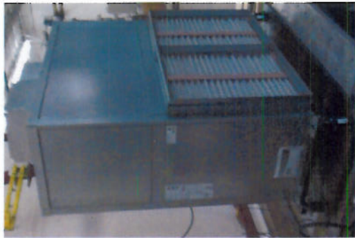
CW40, Base Mounted on AMSR-1C Isolators
