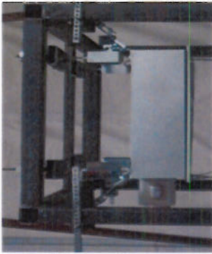
THB02, suspended with HRS-1C hanger boxes
