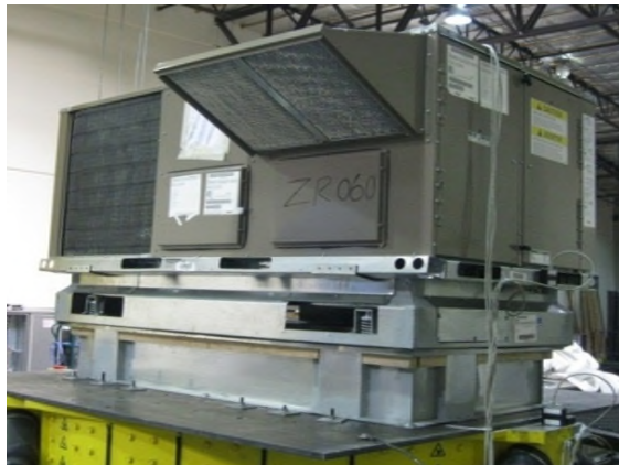
Overall view of UUT-04b
