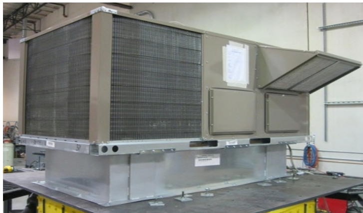
Overall view of UUT-02a
