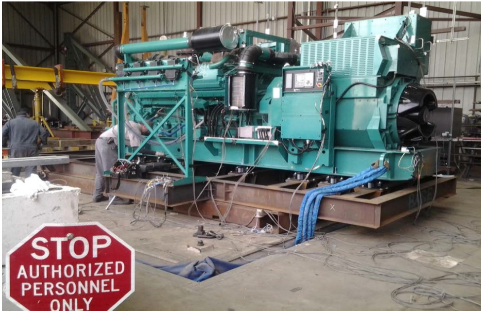
Equipment layout on table. Genset secured to the fixture via (14) CalDyn RJRD-5880 spring isolators.
