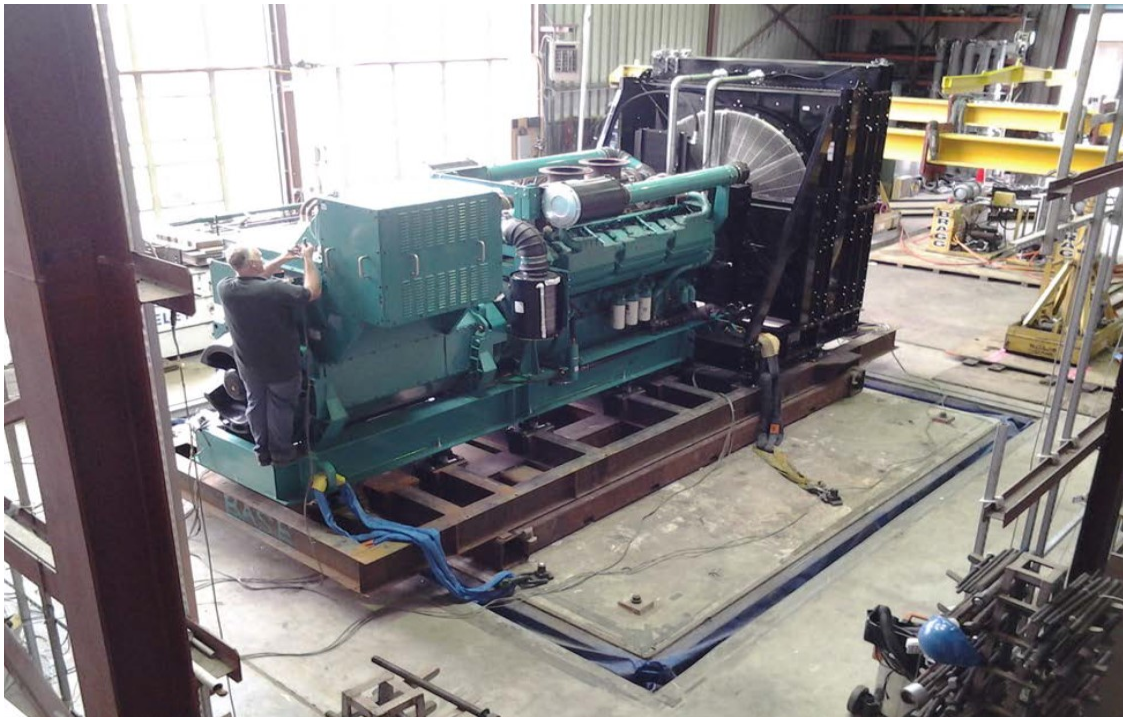
Equipment layout on table. Genset secured to the fixture via (14) California Dynamics Corporation RJRD-5880 spring isolators.
