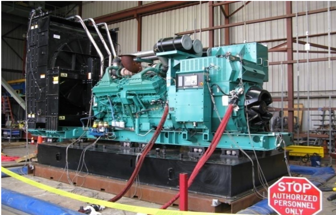
Equipment layout on table. Genset secured to a sub-base tank via (12) VMC M2SSH-1E spring isolators.
