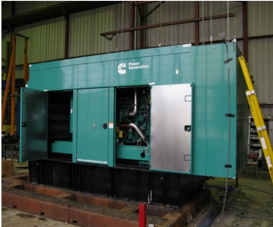
Equipment layout on table. Genset attached to sub-base tank via (4) EBCO 4990-70 duro elastomer isolators. Sub-base tank secured to fixture using (12) 3/4" dia ASTM 325 bolts.
