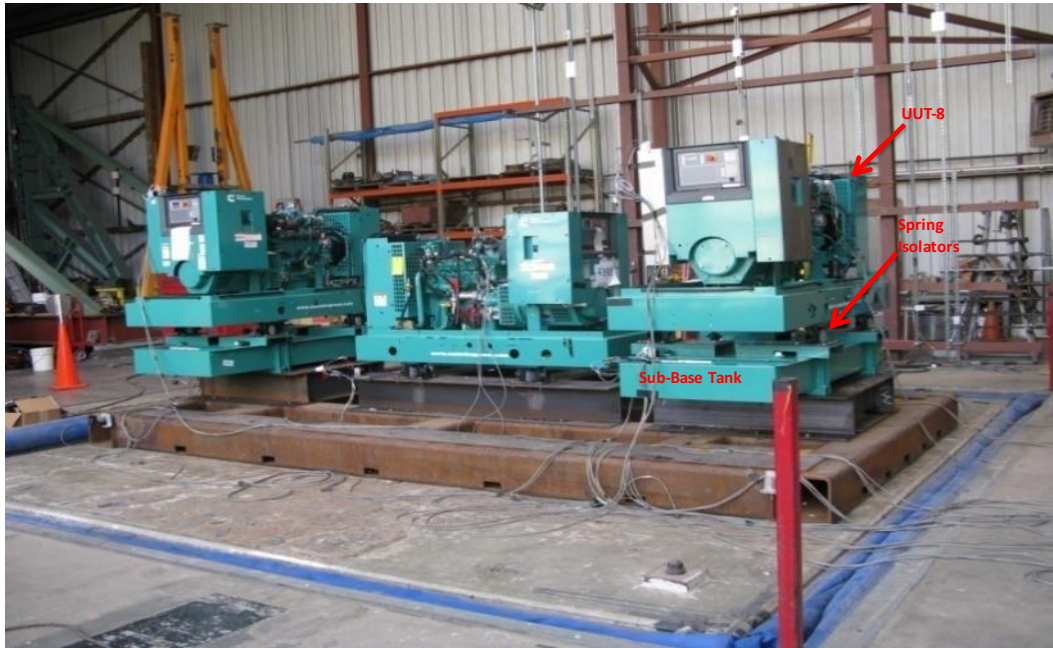
Equipment layout on table. Genset attached to a sub-base tank via (4) Caldyn RJJEQ AE1000 spring isolators. Sub-base tank secured to fixture using (4) 3/4" dia ASTM 325 bolts.
