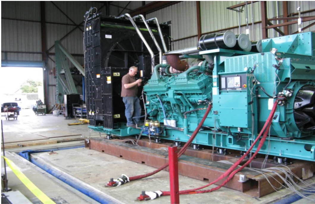
Equipment layout on table. Genset secured to the fixture via (16) CalDyn RJJEQ-D-5880 spring isolators.
