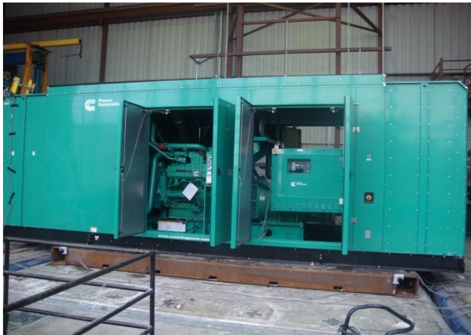
Equipment layout on table. Genset attached to enclosure base via (10) VMC M2SSH-1E-3400N spring isolators. Enclosure base secured to fixture using (12) 3/4" dia SAE Grade 8 bolts.
