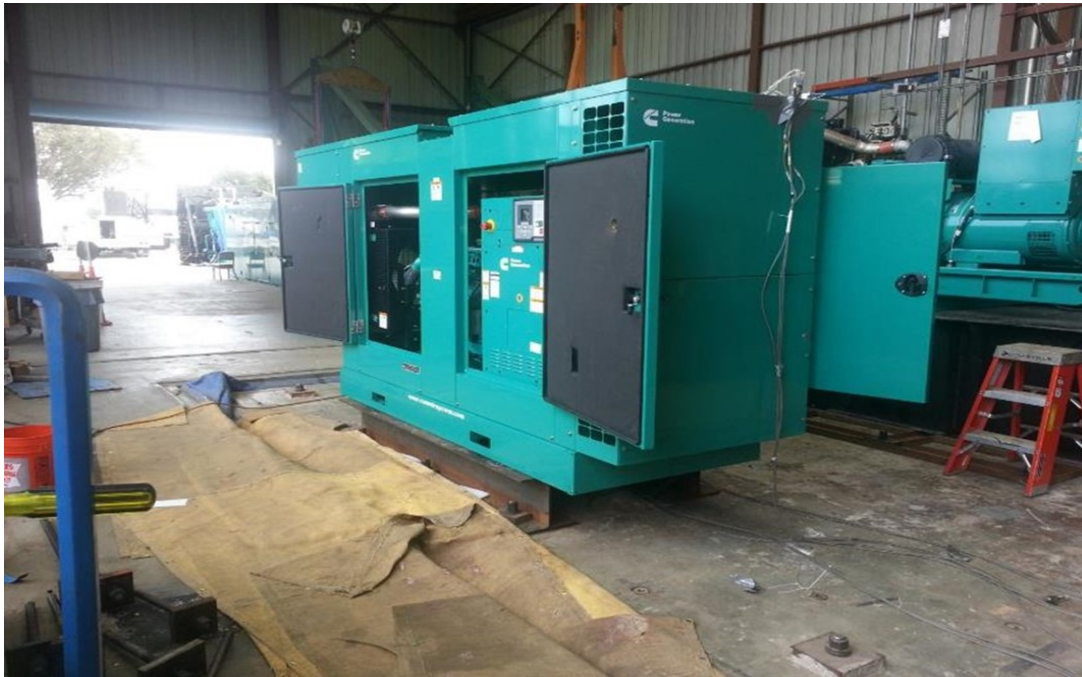
Equipment layout on table. Genset secured to the fixture using (4) 3/4" dia ASTM 325 bolts.
