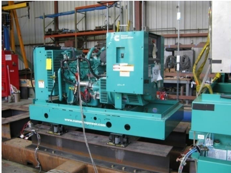
Equipment layout on table. Genset secured to fixture using (4) CalDyn RJJEQ A E1000 spring isolators.
