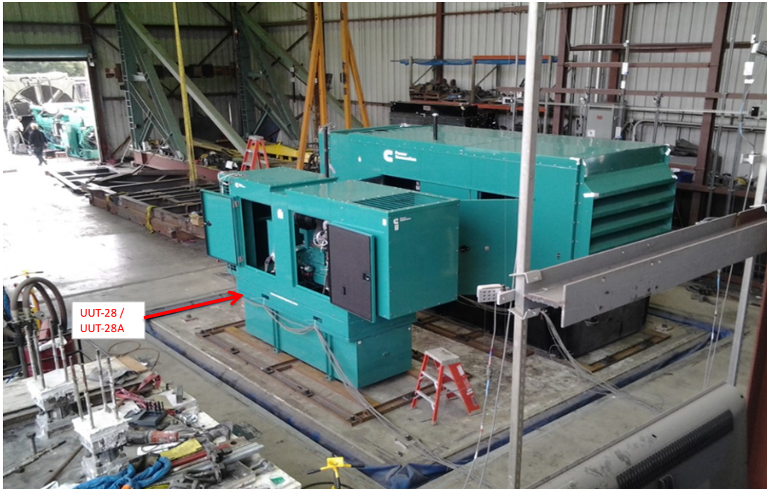
Equipment layout on table. Genset secured to a sub-base tank using (4) 3/4" dia ASTM 325 bolts.
