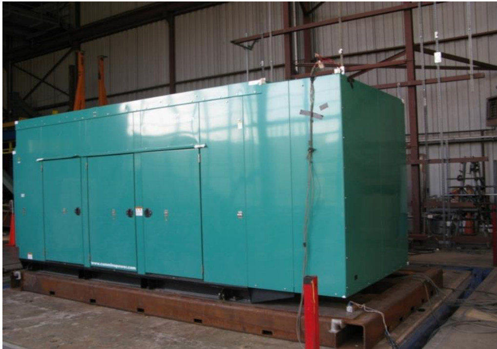
Equipment layout on table. Genset attached to enclosure base via (4) EBCO 4990-70 duro elastomer isolators. Enclosure base secured to fixture using (8) 3/4" dia ASTM 325 bolts.
