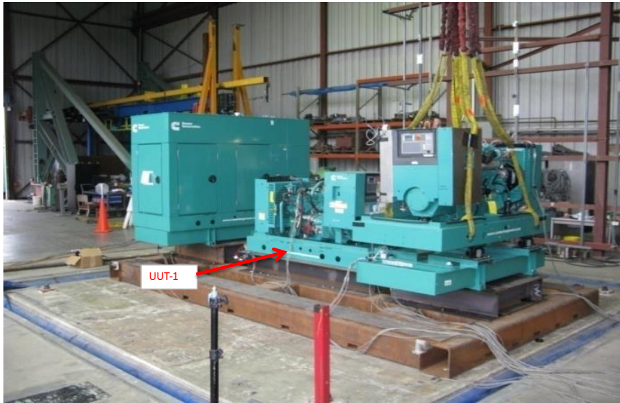
Equipment layout on table. Genset secured to fixture using (4) 3/4" dia ASTM 325 bolts
