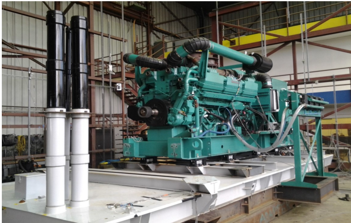
Equipment layout on table. Genset secured to a sub-base tank via (10) VMC M2SSH-1E-6500N spring isolators.
