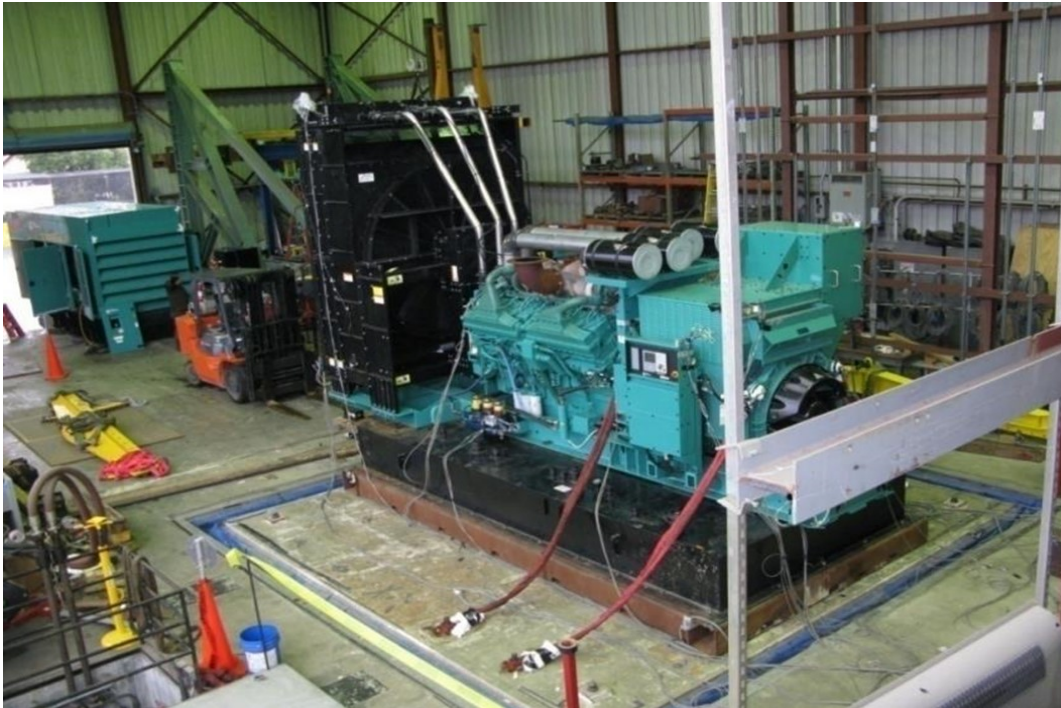
Equipment layout on table. Genset secured to a sub-base tank using (12) 3/4" dia ASTM 325 bolts. Sub-base tank secured to the fixture using (32) 3/4" dia ASTM 325 bolts.
