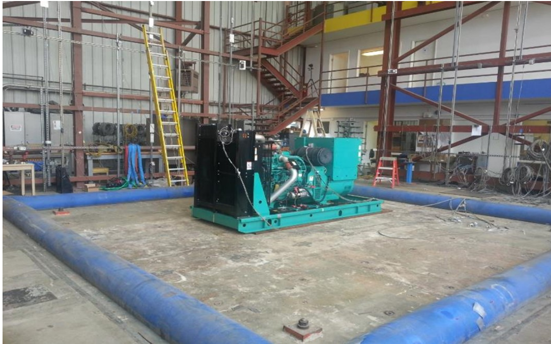
Equipment layout on table. Genset secured to the fixture using (4) 3/4" dia ASTM 325 bolts.
