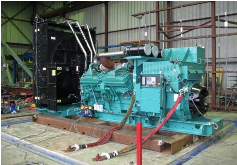
Equipment layout on table. Genset secured to the fixture using (12) 3/4" dia ASTM 325 bolts.
