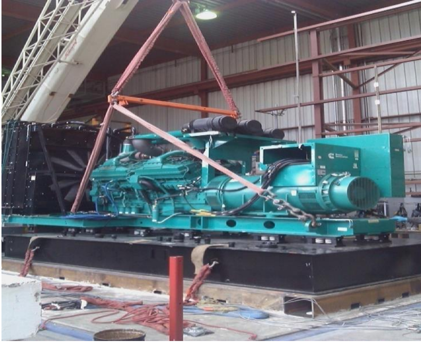
Equipment layout on table. Attached to a sub-base tank via (12) VMC M2SSH-1E spring isolators.
