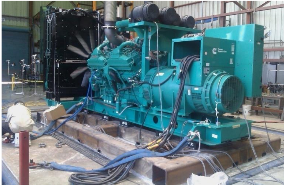
Equipment layout on table. Genset secured to the fixture via (12) VMC M2SSH-1E spring isolators.
