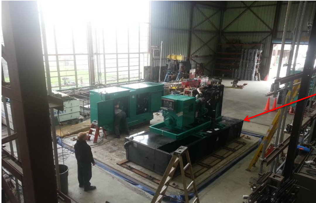
Equipment layout on table. Genset secured to a sub-base tank via (4) EBCO 4990-60 duro elastomer isolators.
