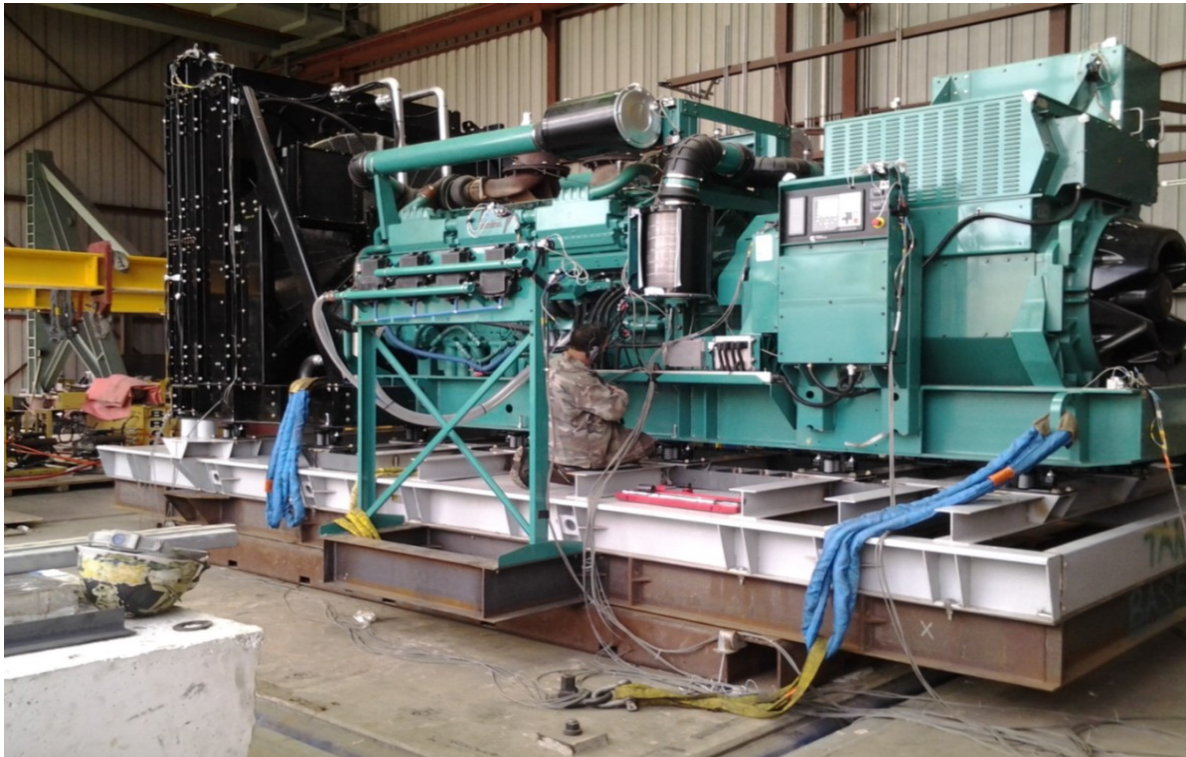
Equipment layout on table. Genset secured to a sub-base tank via (14) CalDyn RJRD-5880 spring isolators.
