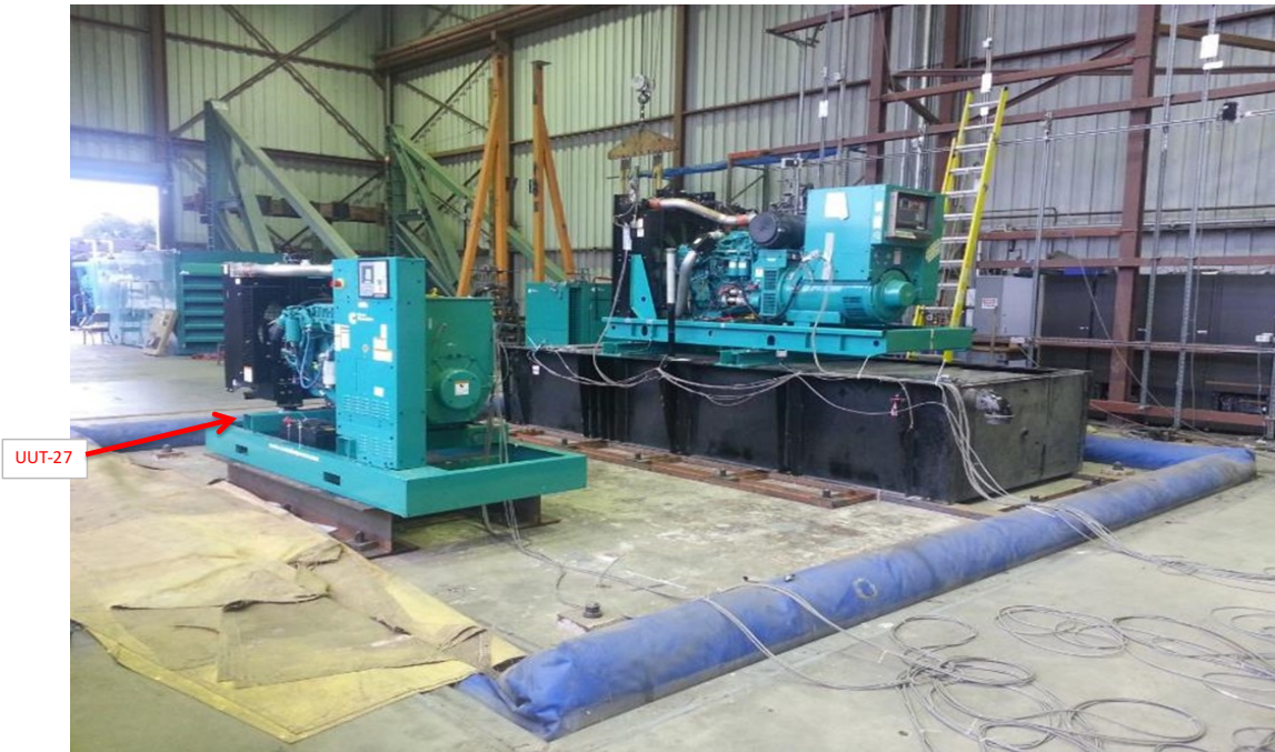
Equipment layout on table. Sub-base tank secured to the fixture using (4) 3/4" dia ASTM 325 bolts.
