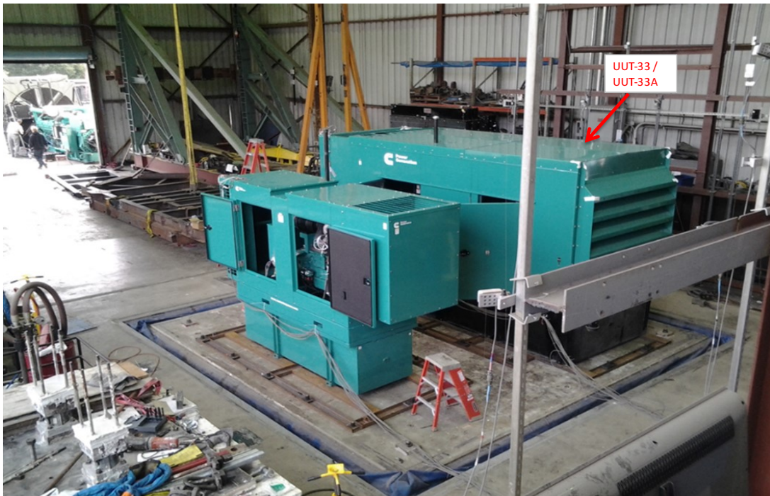
Equipment layout on table. Genset secured to a sub-base tank via (4) EBCO 4990-60 duro elastomer isolators.
