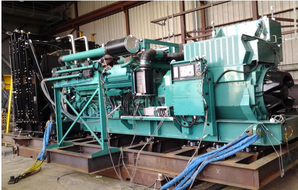
Equipment layout on table. Genset secured to the fixture via (18) CalDyn RJRD-5880 spring isolators.
