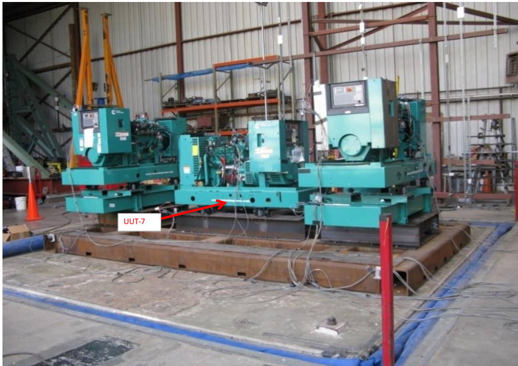
Equipment layout on table. Genset secured to fixture using (4) CalDyn RJJEQ A E1000 spring isolators.
