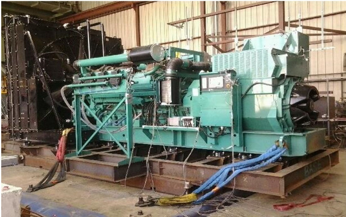
Equipment layout on table. Genset secured to the fixture via (18) CalDyn RJRD-5880 spring isolators.
