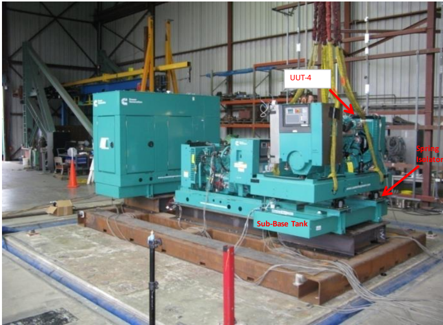
Equipment layout on table. Genset attached to a sub-base tank via (4) Caldyn RJJEQ AE1000 spring isolators. Sub-base tank secured to fixture using (4) 3/4" dia ASTM 325 bolts.
