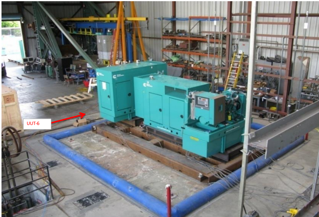
Equipment layout on table. Sub-base tank secured to fixture using (4) 3/4" dia ASTM 325 bolts.
