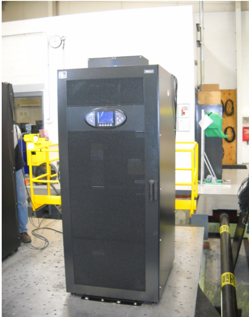
Figure 3: UUT-8 45kVA UPS Attachment Method: hard-mount - 1/2" dia bolts to table, angle brackets by Liebert
