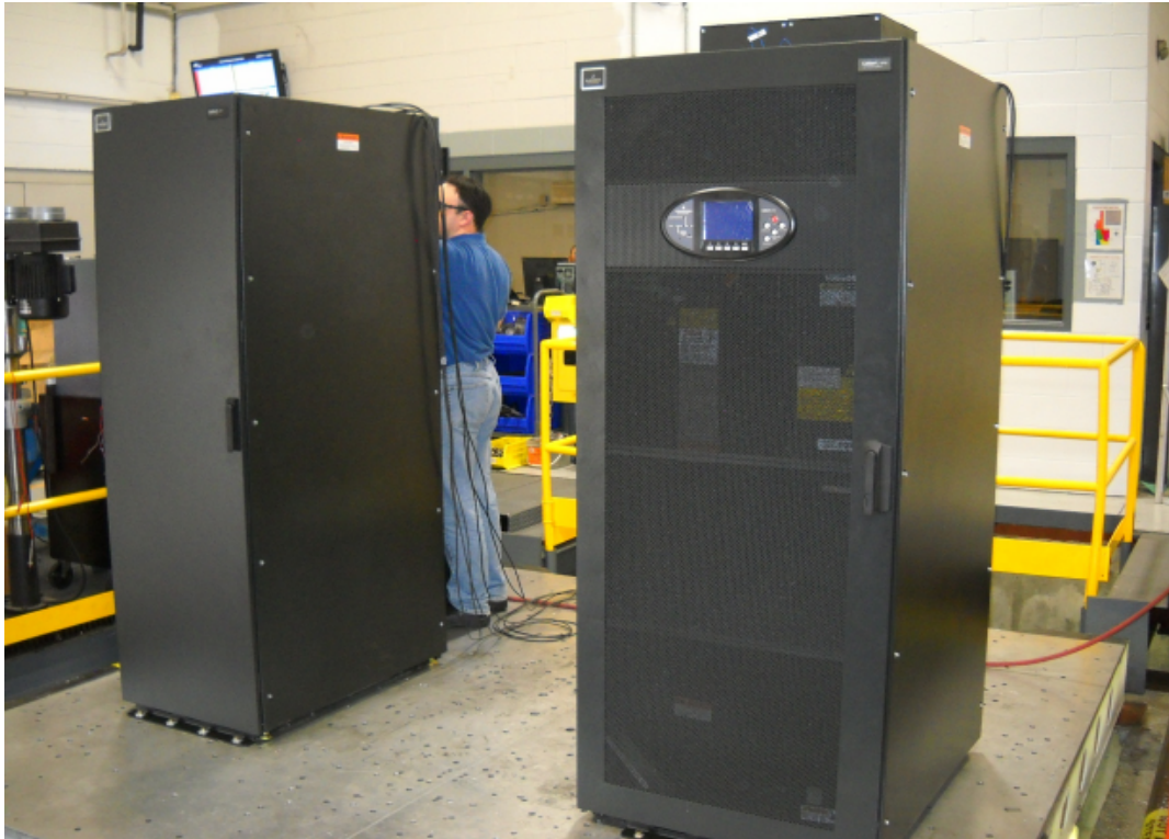
Figure 1: UUT-7 15kVA UPS (right) and UUT-11 90kVA BDC (left) Attachment Method: hard-mount - 1/2" dia bolts to table, angle brackets by Liebert
