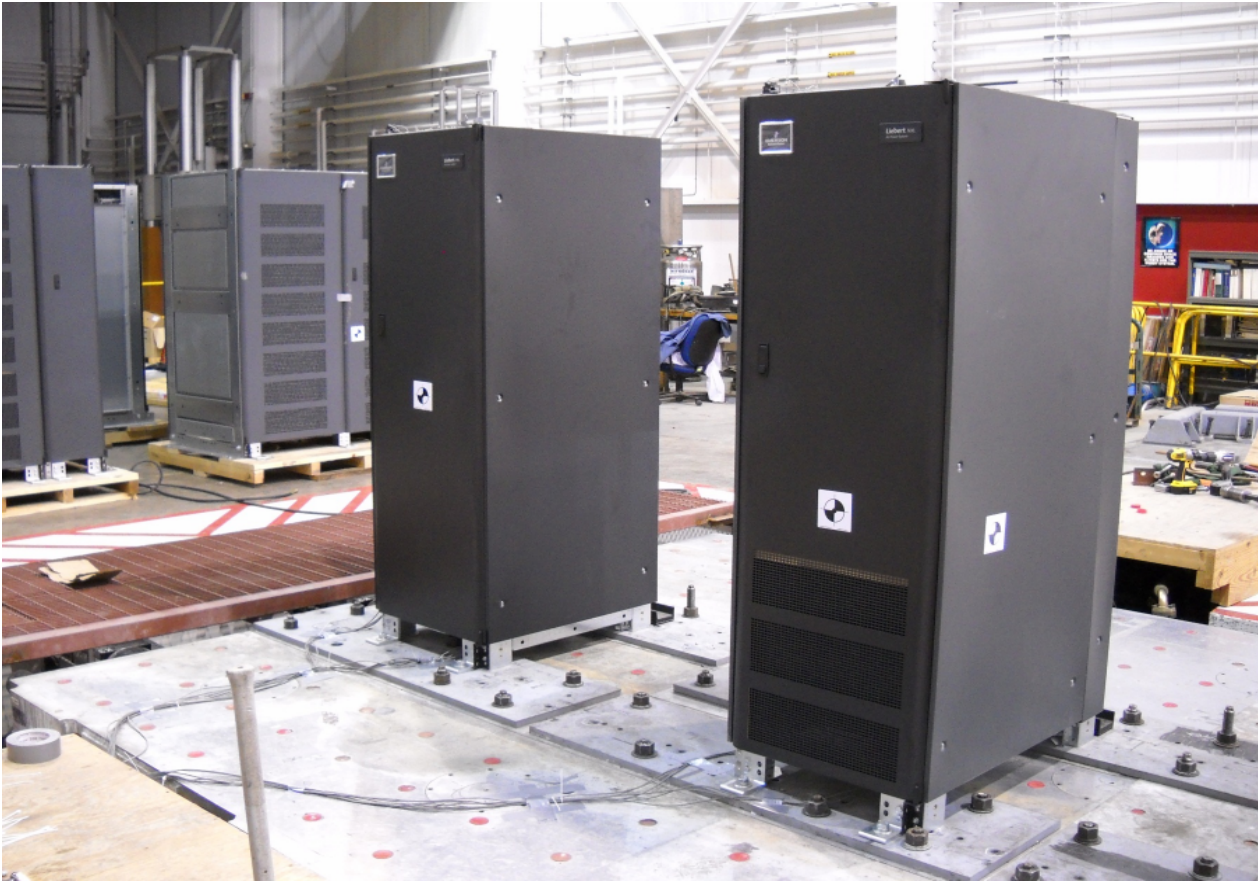
Figure 6: UUT-7 250kVA MBC (left) and UUT-8 500kVA MBC (right) Attachment Method: hard-mount - (4)-3/4" dia bolts each to table, angle brackets by Liebert
