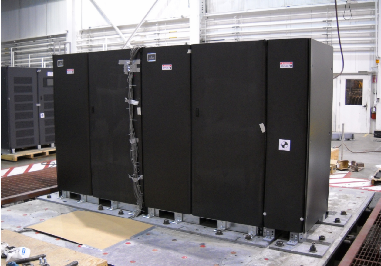
Figure 4: UUT-5 12V Top Terminal Battery Cabinet (UUT-9 Junction Cabinet on right side) Attachment Method: hard-mount - (20)-3/4"dia bolts to table, angle brackets by Liebert
