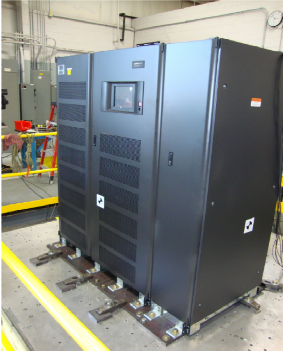
Figure 1: UUT-1 250kVA UPS Attachment Method: hard-mount - (14)-3/4"dia bolts to table, angle brackets by Liebert
