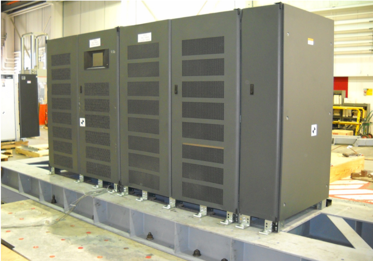
Figure 2: UUT-3 750kVA UPS Attachment Method: hard-mount - (22)-3/4"dia bolts to fixture, angle brackets by Liebert
