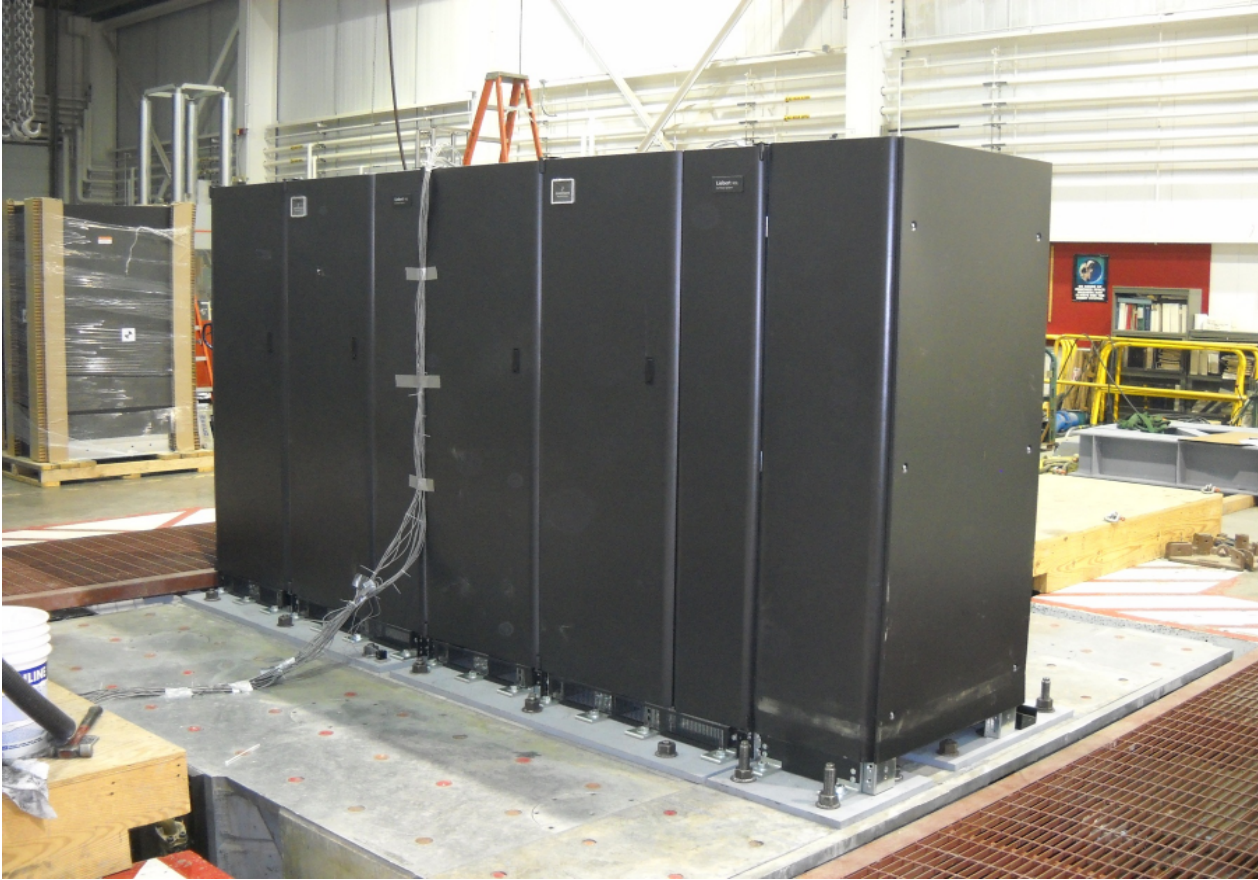
Figure 5: UUT-6 16V Front Terminal Battery Cabinet (UUT-10 Junction Cabinet on right side) Attachment Method: hard-mount - (32)-3/4" dia bolts to table, angle brackets by Liebert
