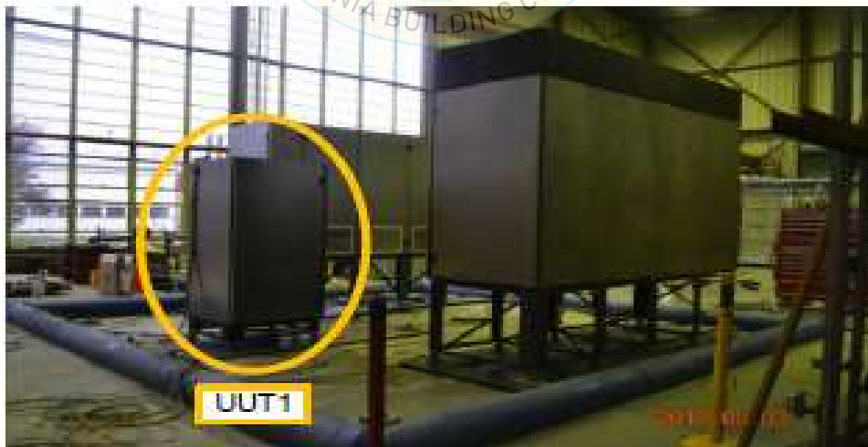
All units were filled with contents and maintained structural integrity and functionality after AC156 test.
