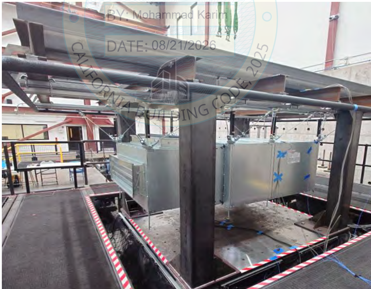
Overall view of UUT-15A.
