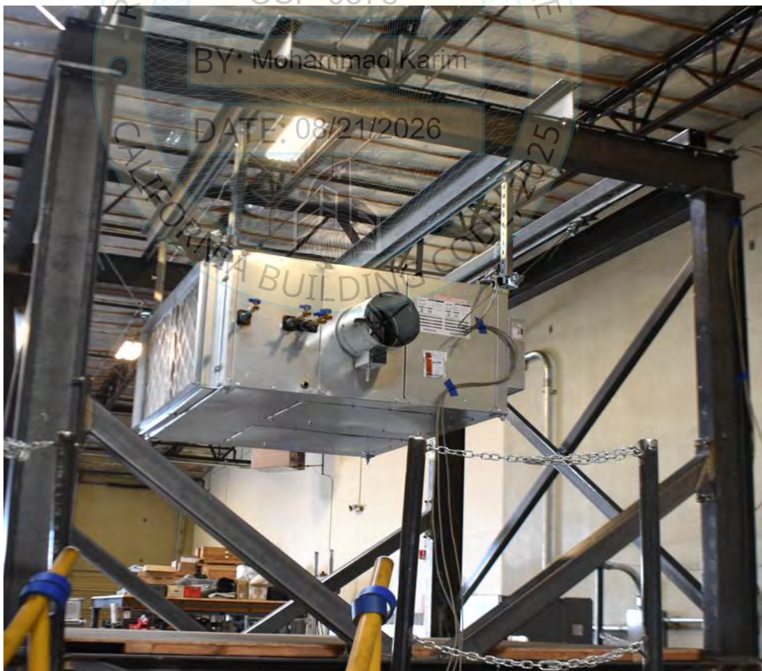
Overall view of UUT-13A.
