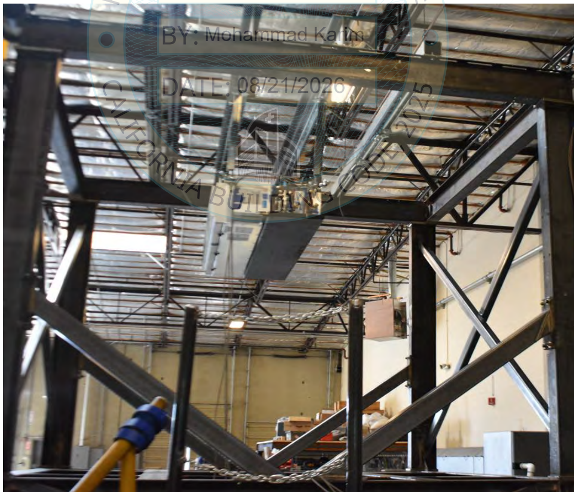
Overall view of UUT-10A.
