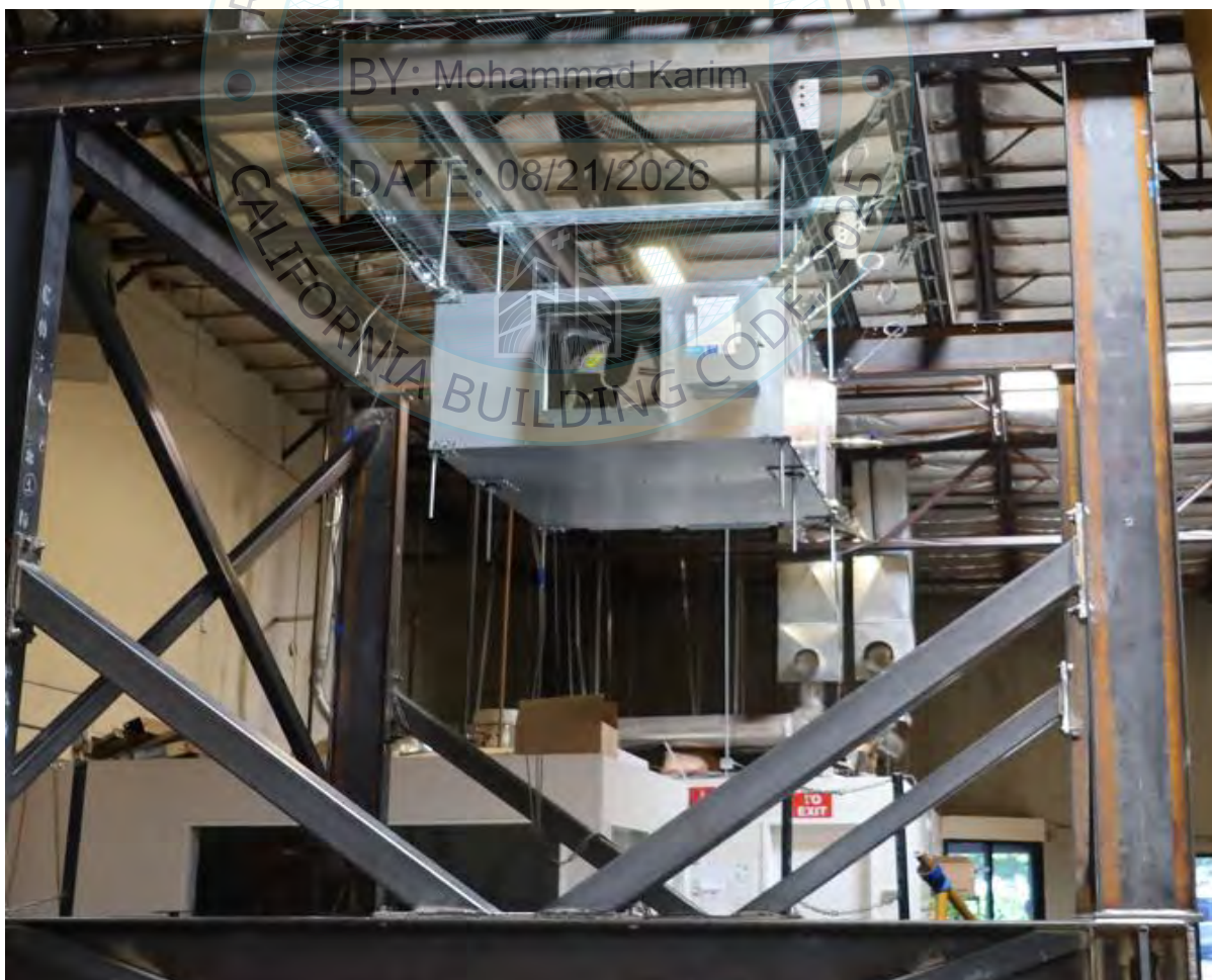
Overall view of UUT-14A.
