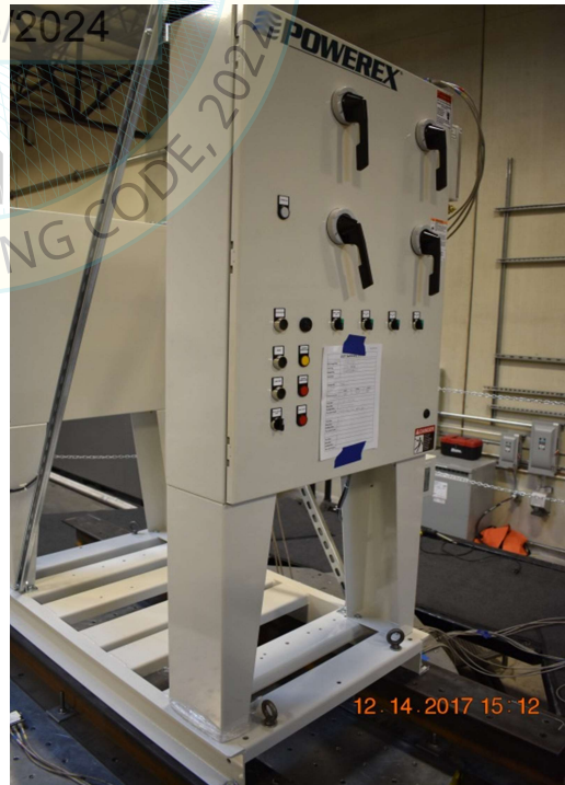
UUT14b - quadruplex panel
