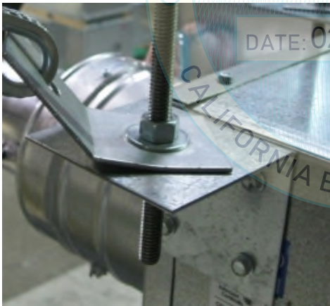
Photograph showing typical angle bracket mounting for UUT15.
