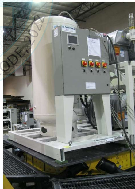
UUT2, view from left
