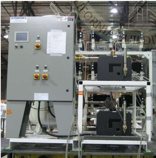
UUT3, view from front
