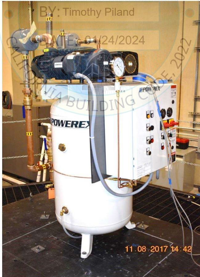
UUT21 Overall View
