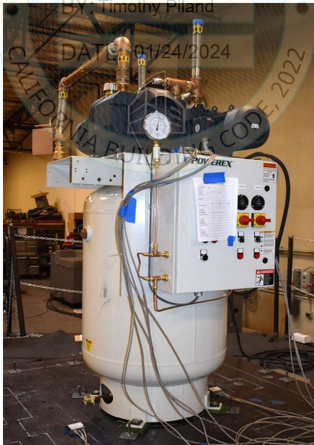
UUT23 Overall View
