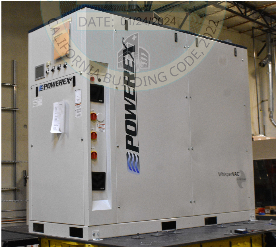
UUT38 Overall View
