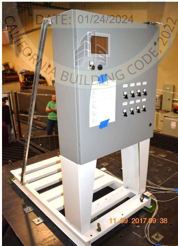
UUT13 Overall View
