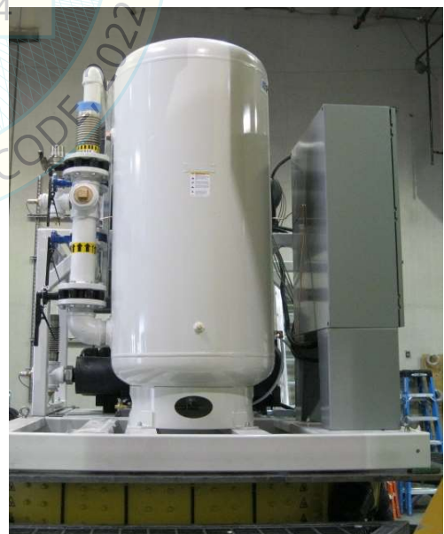
UUT4, view from left
