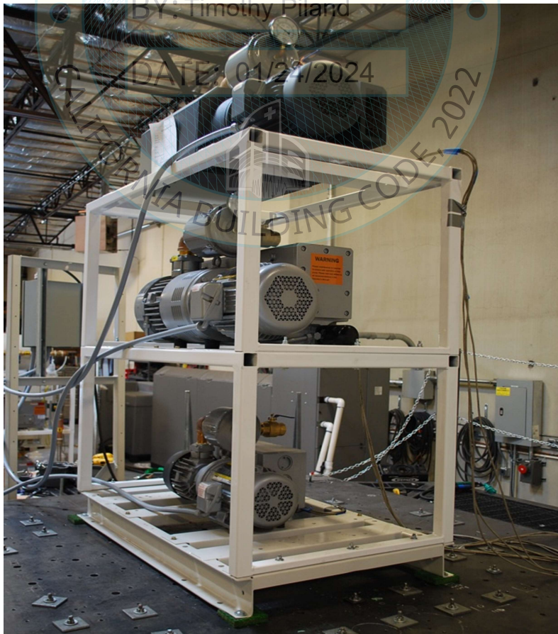
UUT8 Overall View
