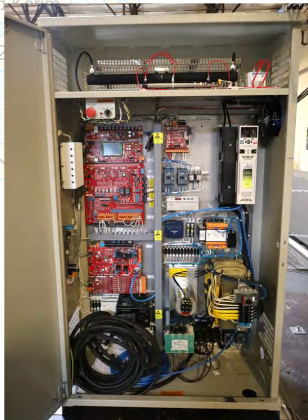
UUT19 interior view
