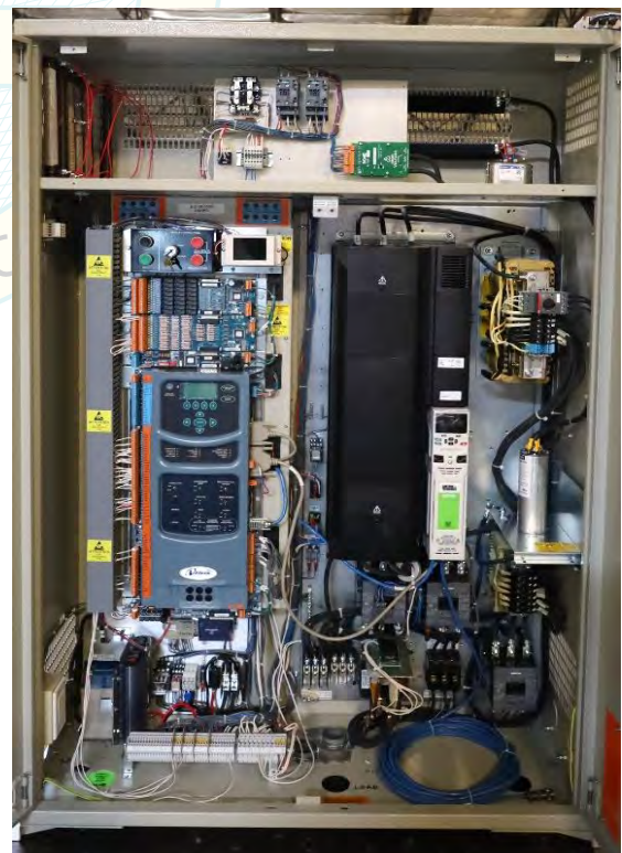
UUT18 interior view
