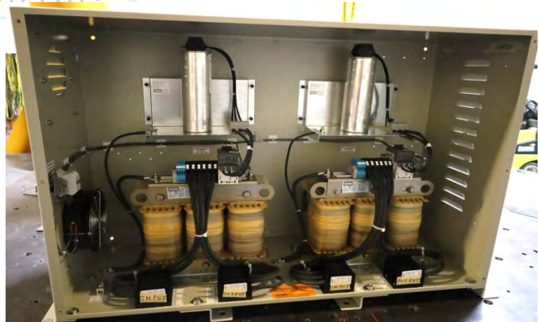
UUT20 interior view
