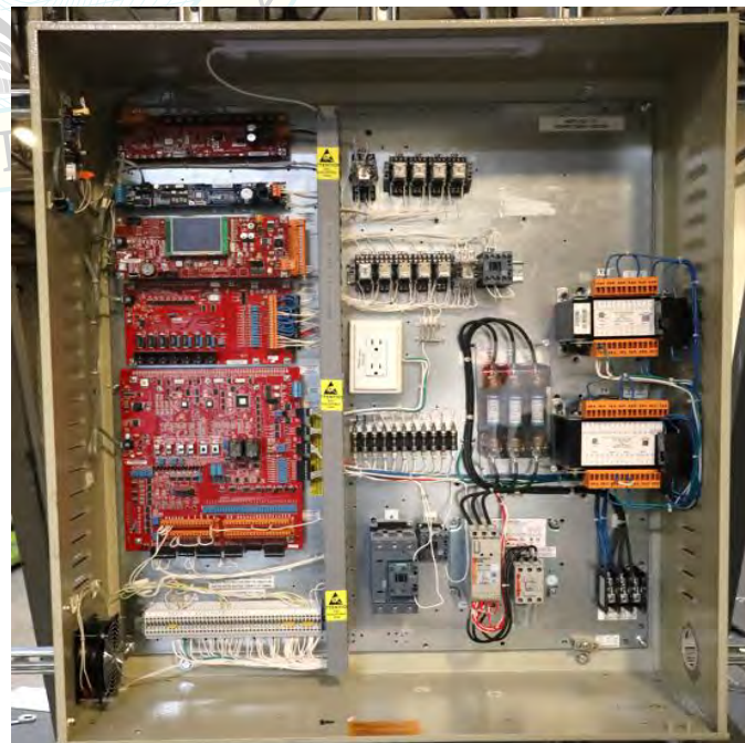
UUT17b interior view
