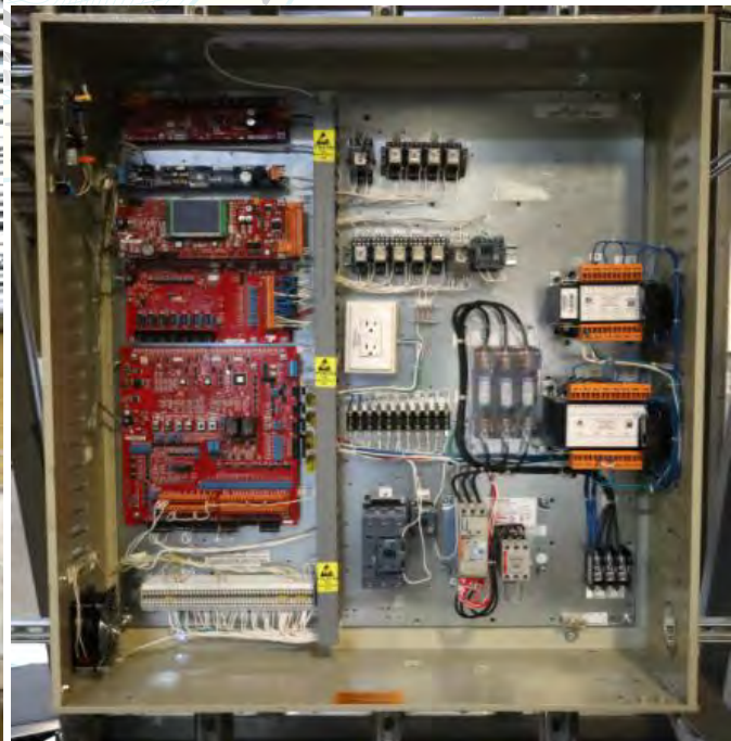
UUT17a interior view
