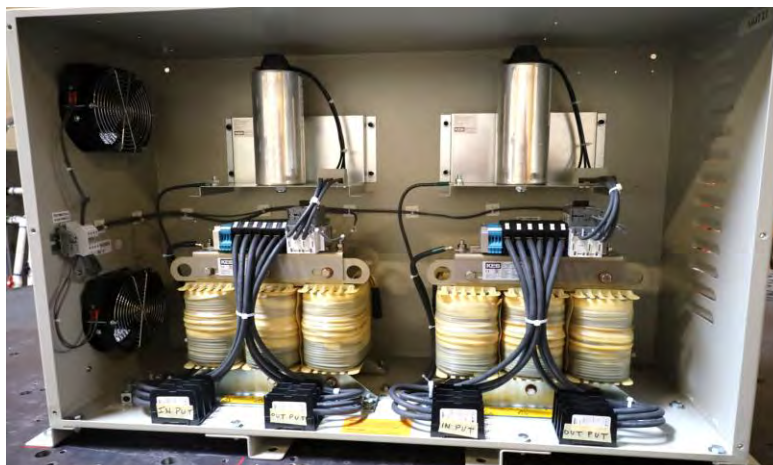
UUT21 interior view
