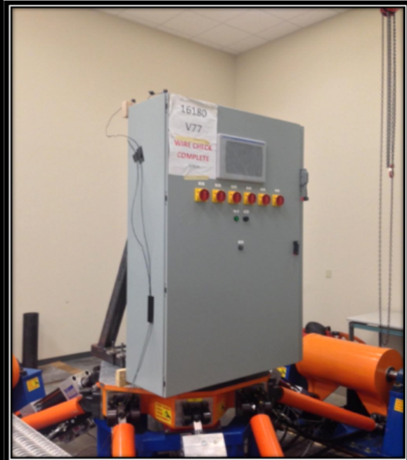
All units were filled with contents and maintained structural integrity and functionality
