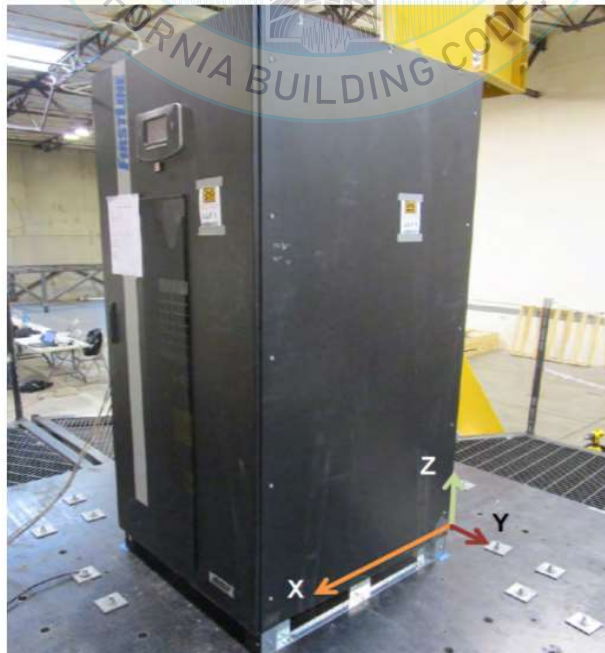
All units were filled with contents and maintained structural integrity and functionality after AC-156 test.
