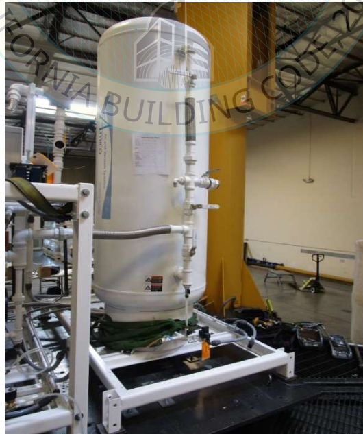
UUT2B Overall View
