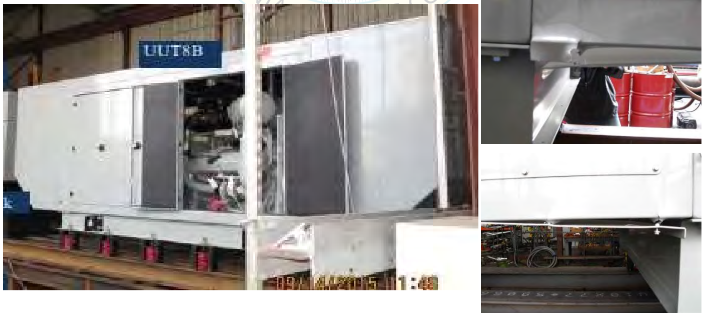
All units were filled with contents and maintained structural integrity and functionality after AC-156 test.
