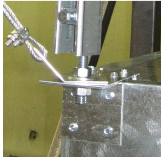
Photograph showing typical mounting for UUT23, UUT26.
