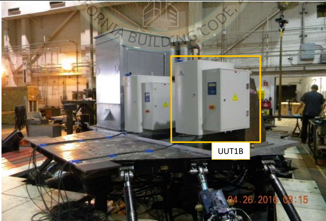
Overall view of UUT1B.1 (Dry)
