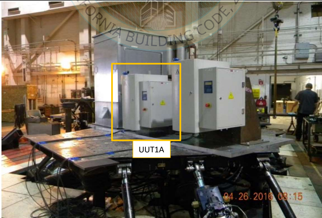
Overall view of UUT1A.1 (Dry)
