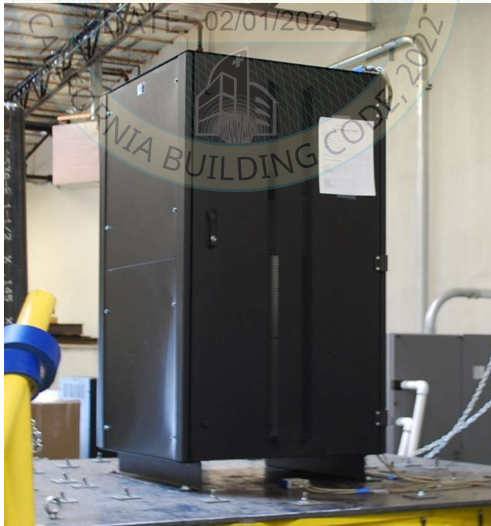
UUT4 Overall View
