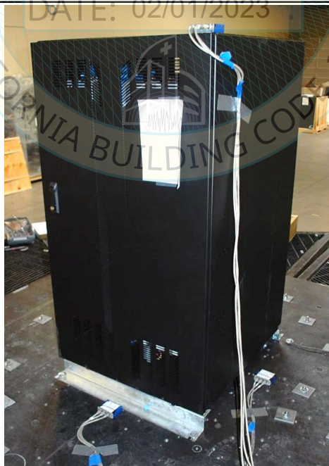
UUT11 Overall View
