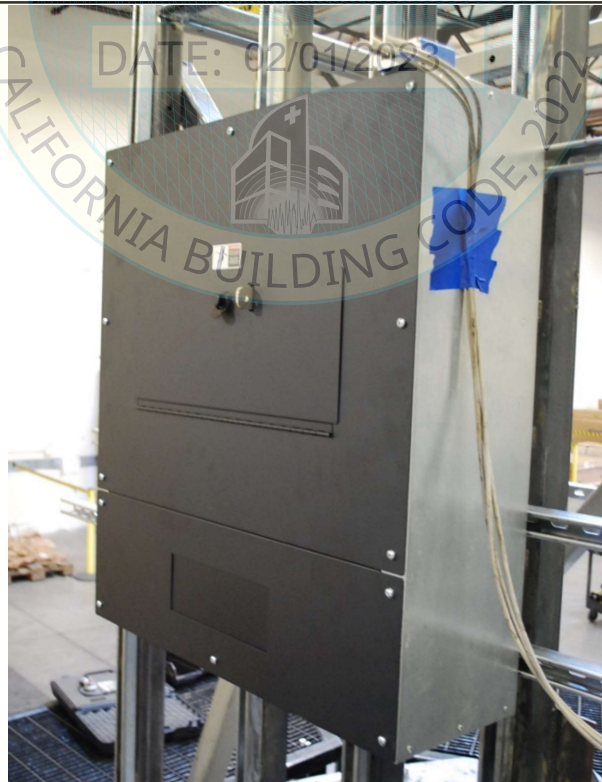
UUT1 Overall View
