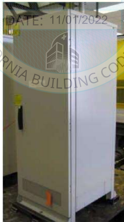
Overall view of UUT-2B
