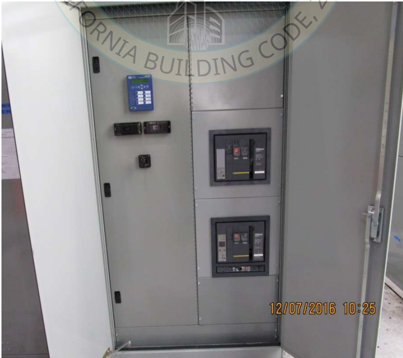
All units were filled with contents and maintained structural integrity and functionality after AC-156 test.
