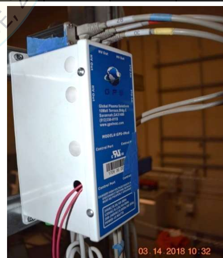
Figure 3. Close up overall view of UUT-03a,b
