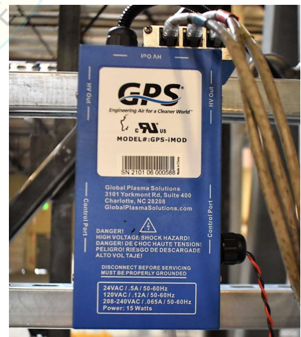
Figure 3. Close up overall view of UUT-07a,b
