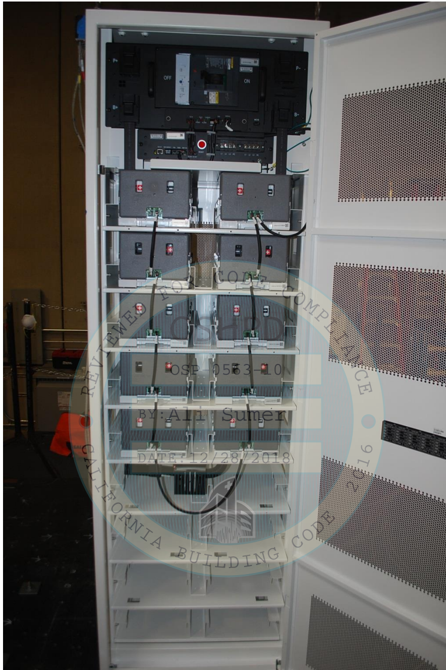
Figure C.8. UUT1a interior view, pre-test
