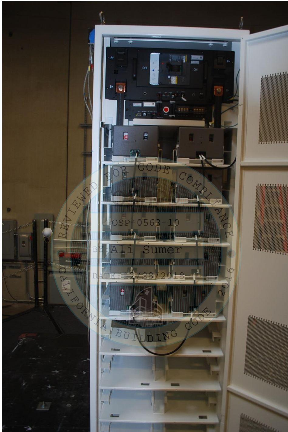
Figure C.10. UUT1a interior view, post-test
