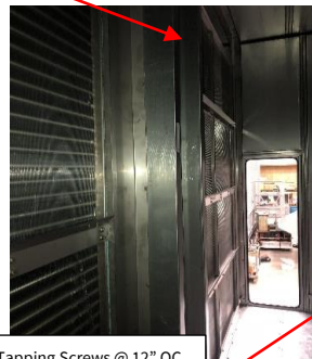
#12-3/4" Self Tapping Screws @ 12" OC Along Length of Blankoff and (5) Self Tapping Screws in Base and Ceiling Panel (Typical)
