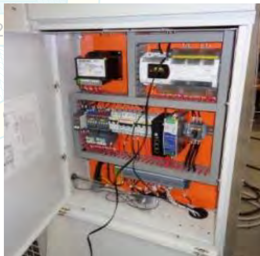
UUT-01 Interior View
