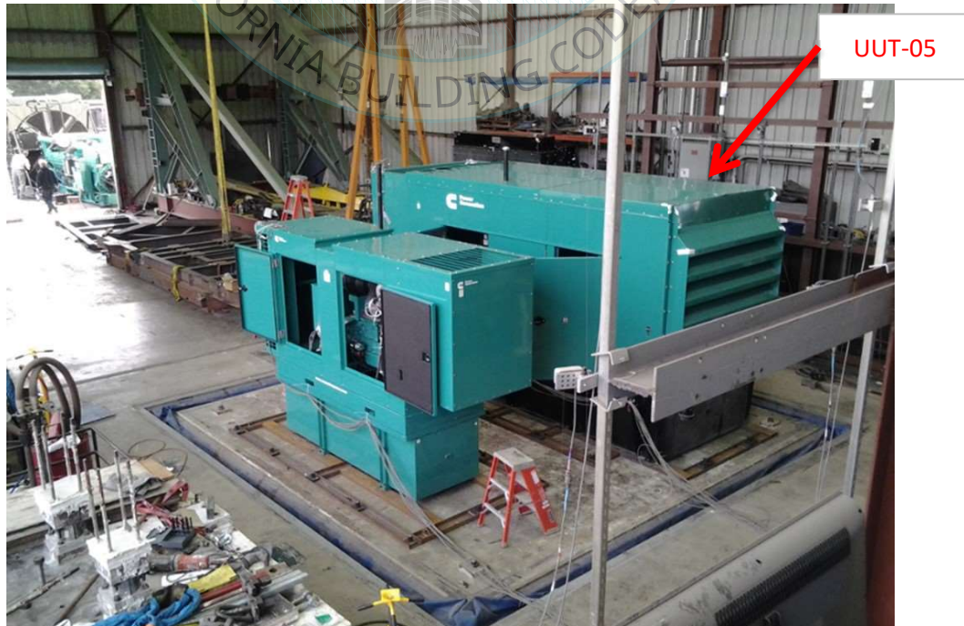
All units were filled with contents and maintained structural integrity and functionality after AC-156 test.
