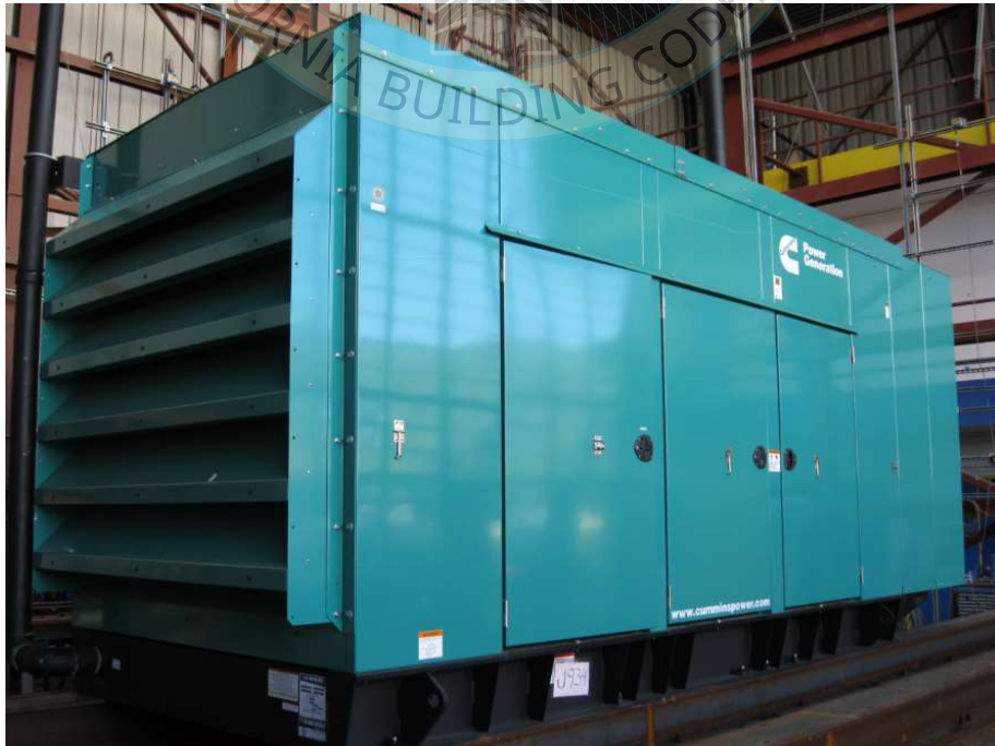
All units were filled with contents and maintained structural integrity and functionality after AC-156 test.
