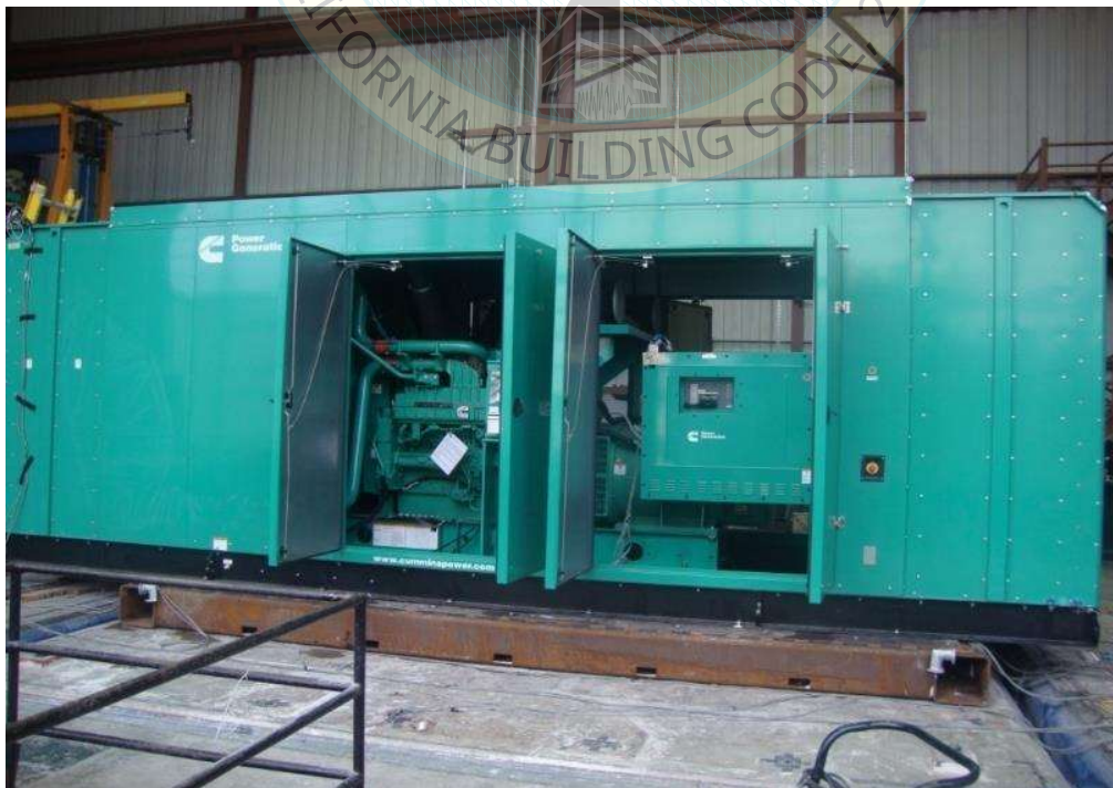
All units were filled with contents and maintained structural integrity and functionality after AC-156 test.
