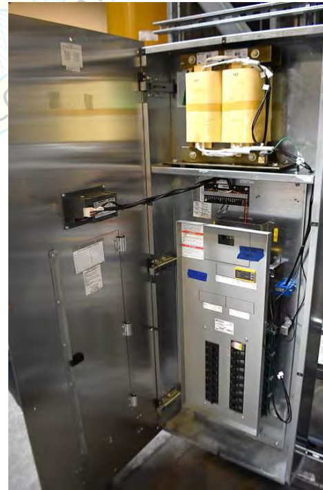
UUT6 Interior View
