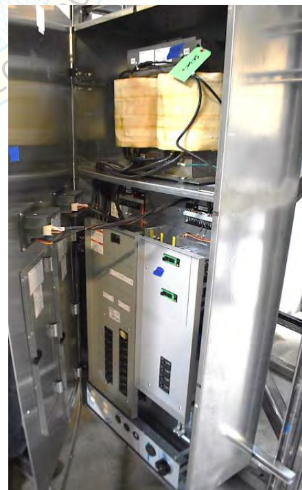
UUT7 Interior View
