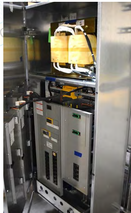
UUT8 Interior View
