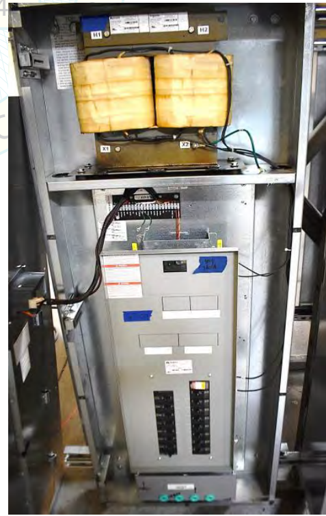
UUT5 Interior View
