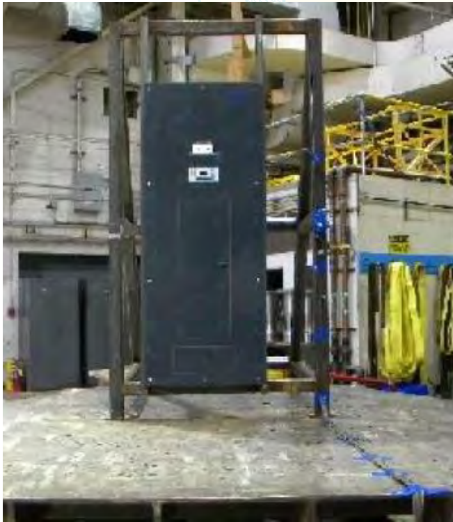
UUT1B Front View
