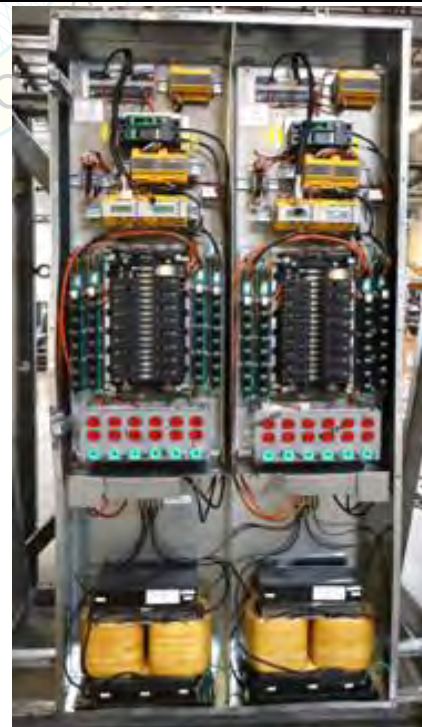
UUT-10 Interior View
