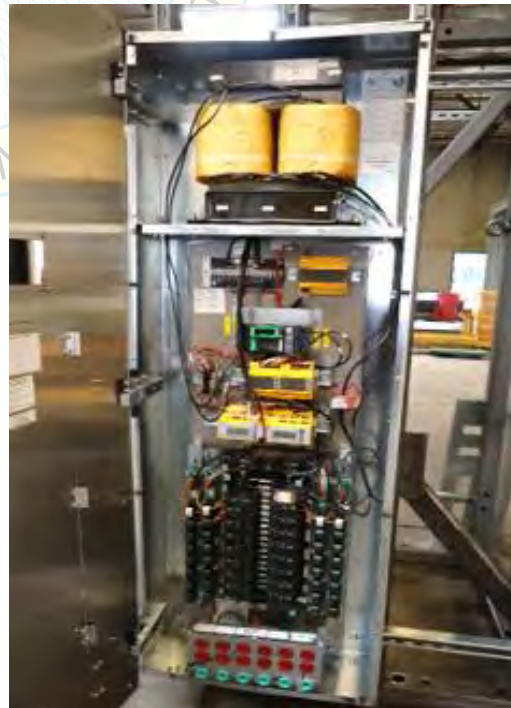
UUT-09 Interior view
