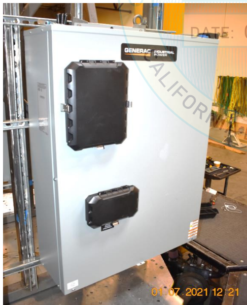
Figure 1. UUT4 Exterior View
