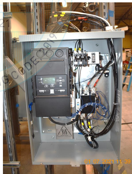
Figure 2. UUT1 Interior View
