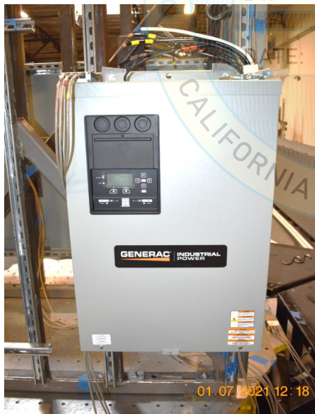
Figure 1. UUT1 Exterior View
