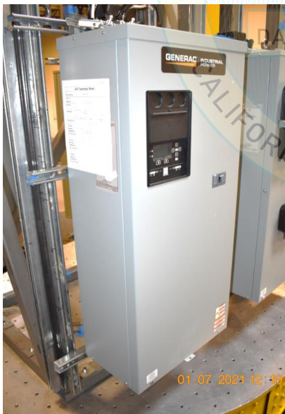
Figure 1. UUT3 Exterior View
