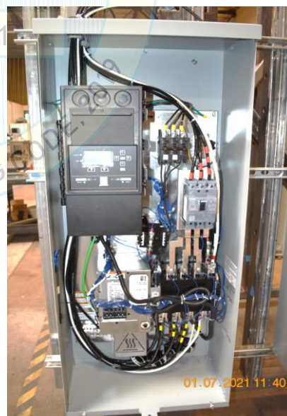
Figure 2. UUT3 Interior View
