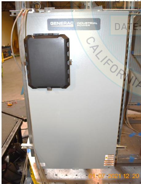
Figure 1. UUT2 Exterior View
