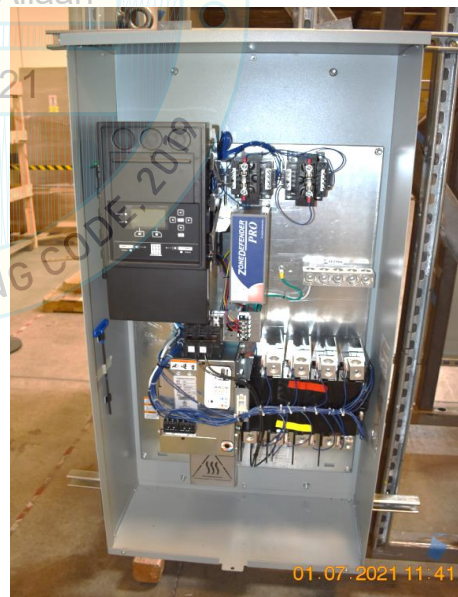
Figure 2. UUT2 Interior View
