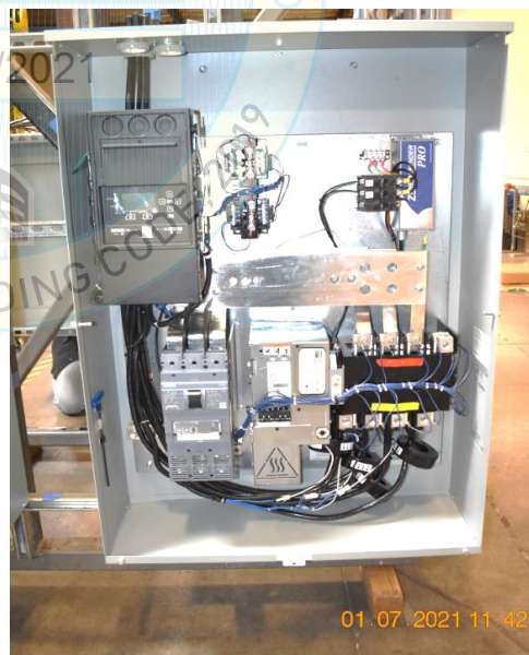
Figure 2. UUT4 Interior View
