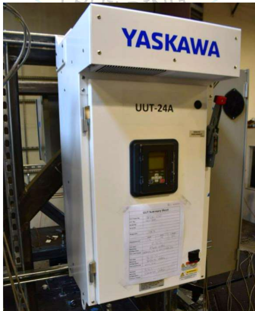
All units were filled with contents and maintained structural integrity and functionality after AC-156 test.
