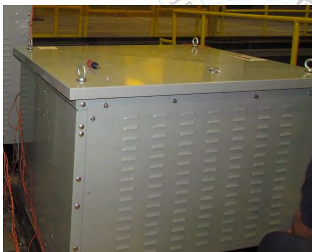
UUT-7 overall view.
