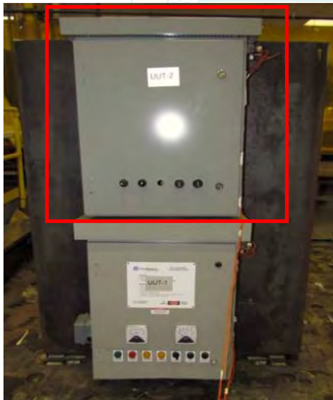
UUT-2 overall view.
