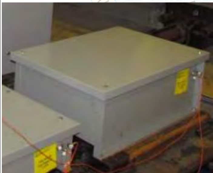
UUT-6 overall view.
