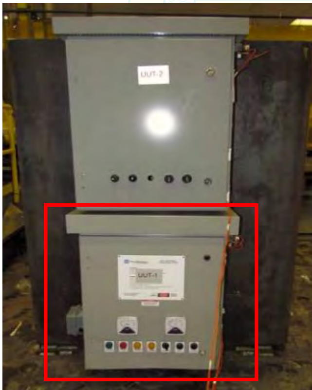
UUT-1 overall view.
