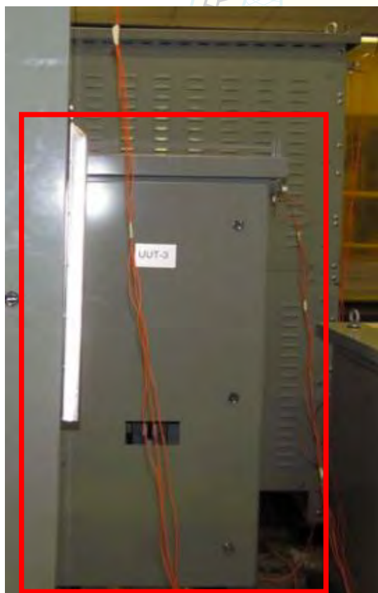
UUT-3 overall view.
