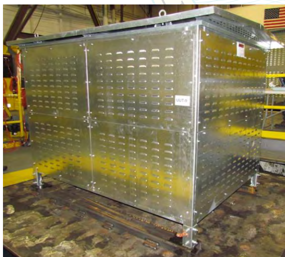
UUT-9 overall view.
