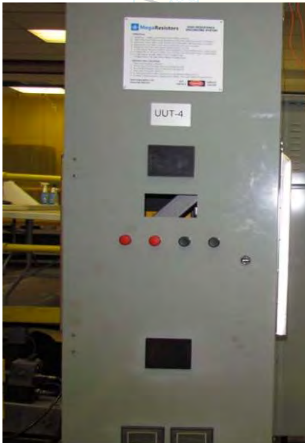
UUT-4 overall view.
