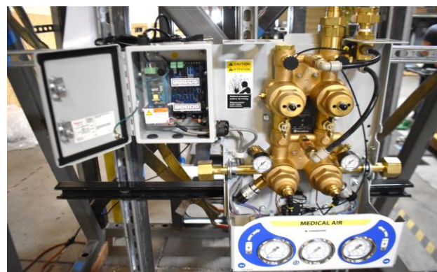
Figure 2. Overall interior view of UUT-1
