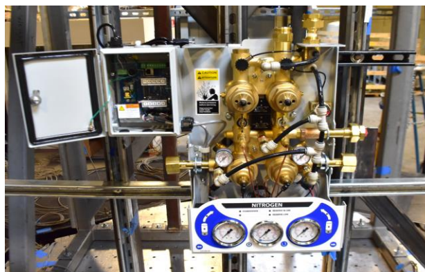
Figure 2. Overall interior view of UUT-2
