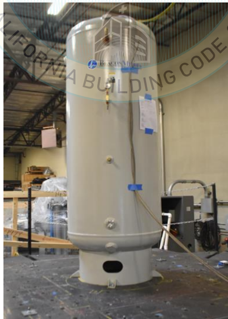
Figure 1. Overall view of UUT-1c
