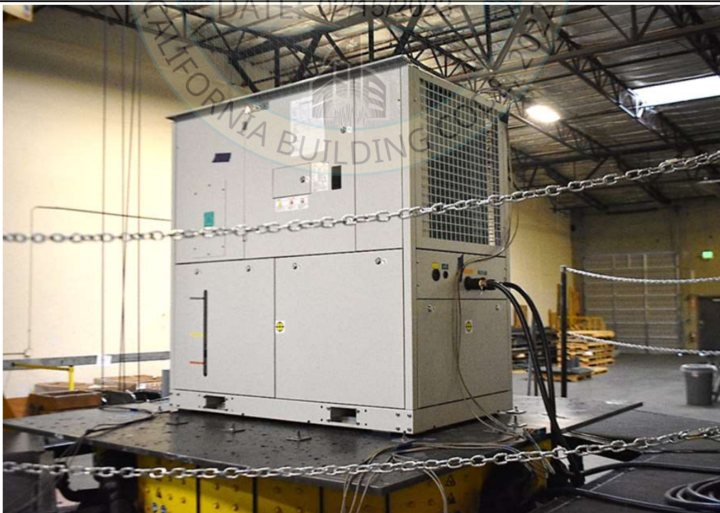
UUT-01 Overall View
