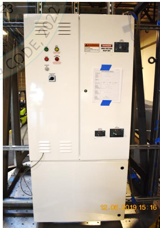
Figure 2. Photograph of UUT-02
