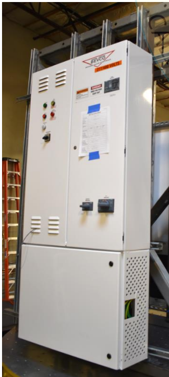
Figure 1. Photograph of UUT-01
